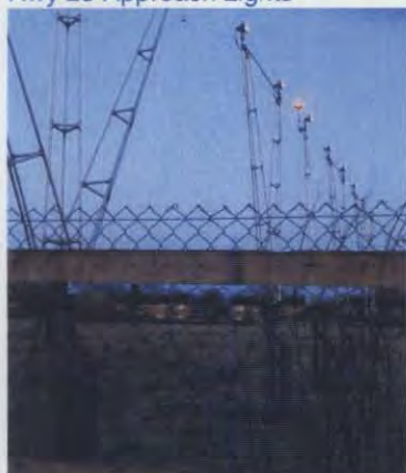
Rwy 25 Approach Lights
