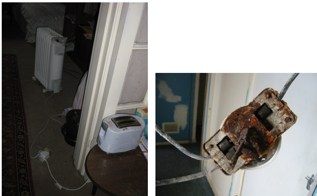
Figure 3.5: Examples of inadequate electrical safety which increase the risk of fire in homes
