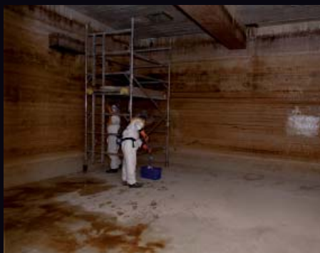
It was 40 years before workers were able to access the concrete External Active Sludge Tanks
