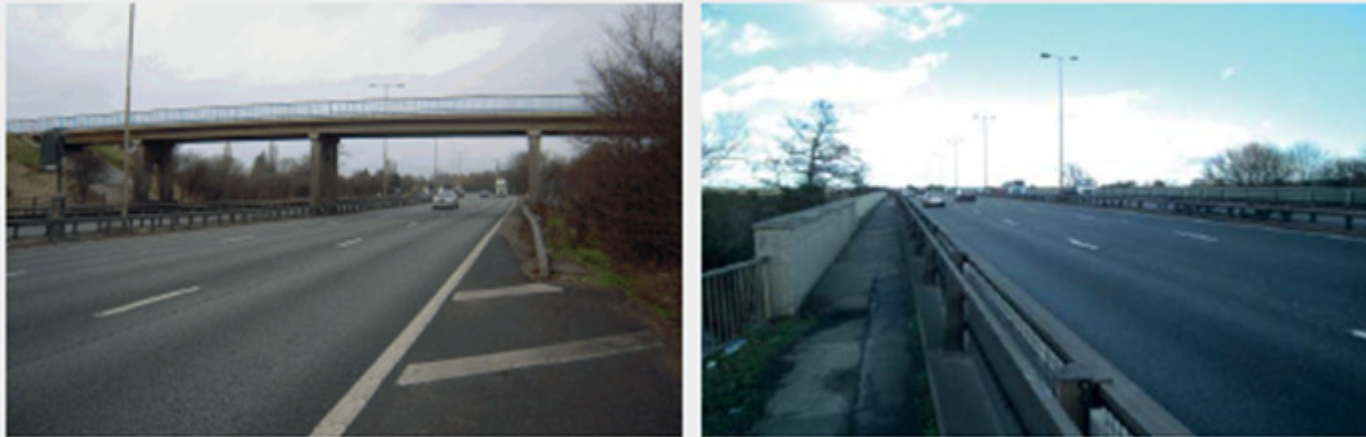
Hard Shoulder Discontinuities Preventing Widening
