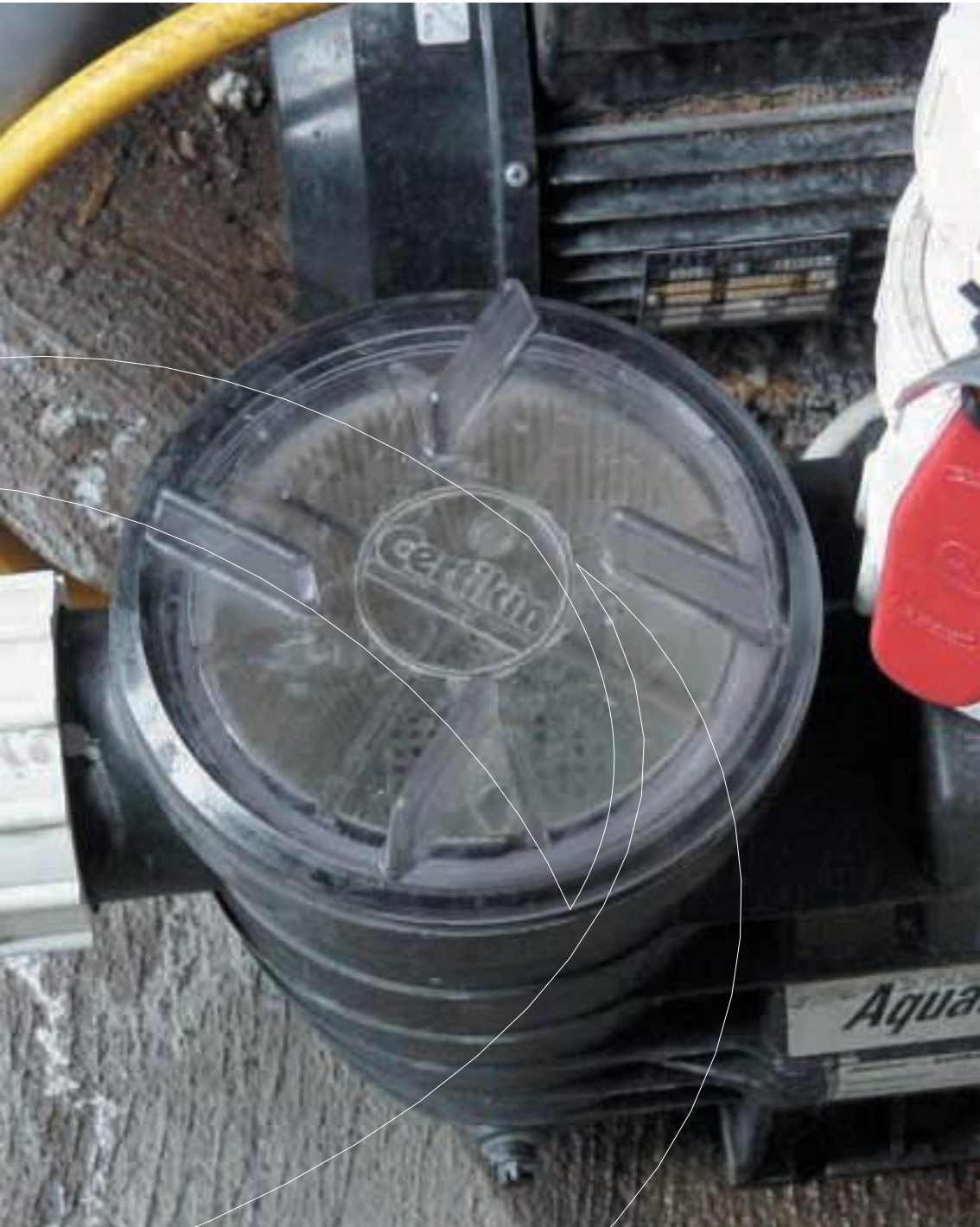
Water pump strainer – needs inspection daily and cleaning if necessary
