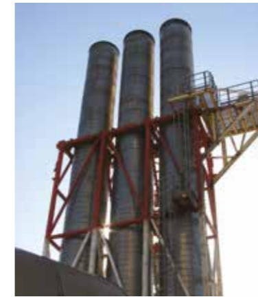
Power generation package exhaust stacks
