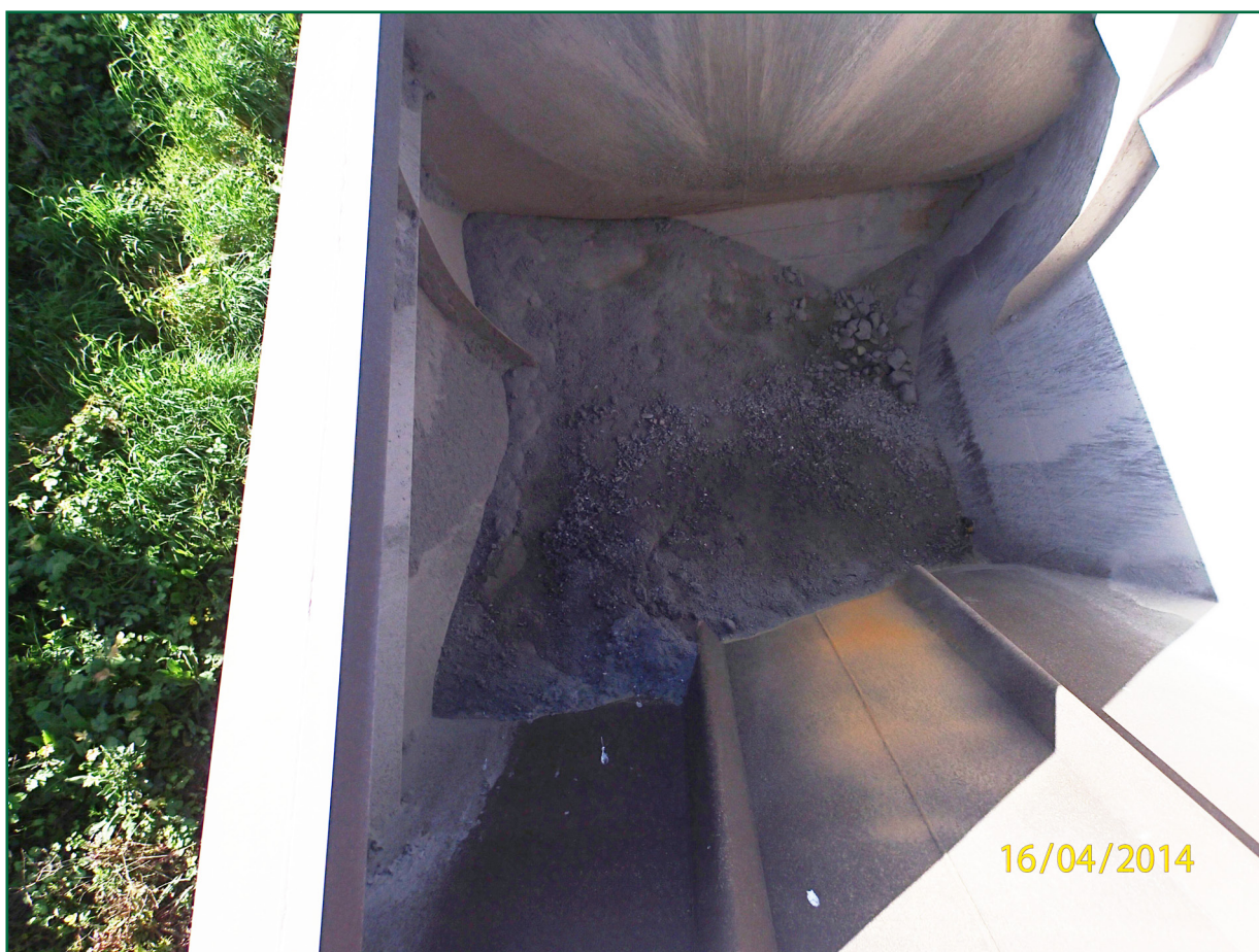
Figure 17: Retained material in the wagon (after derailment)
