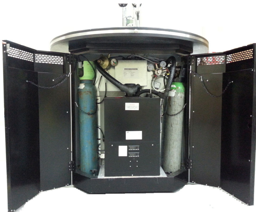
Figure 4 - Photographic back view of inside of cabinet "Dry Side"
