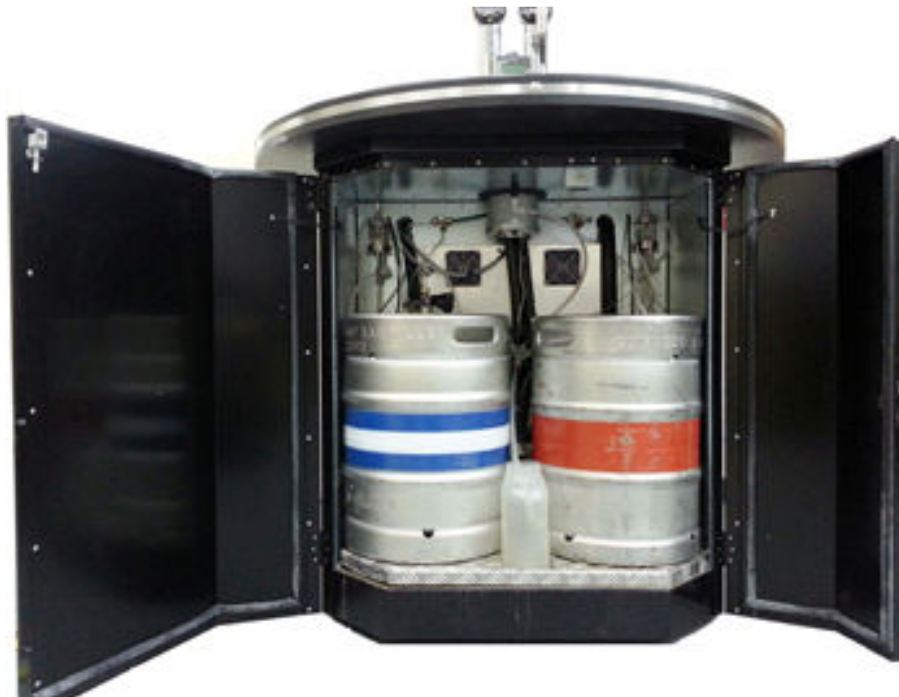
Figure 3 - Photographic front view of inside of cabinet "Wet Side"
