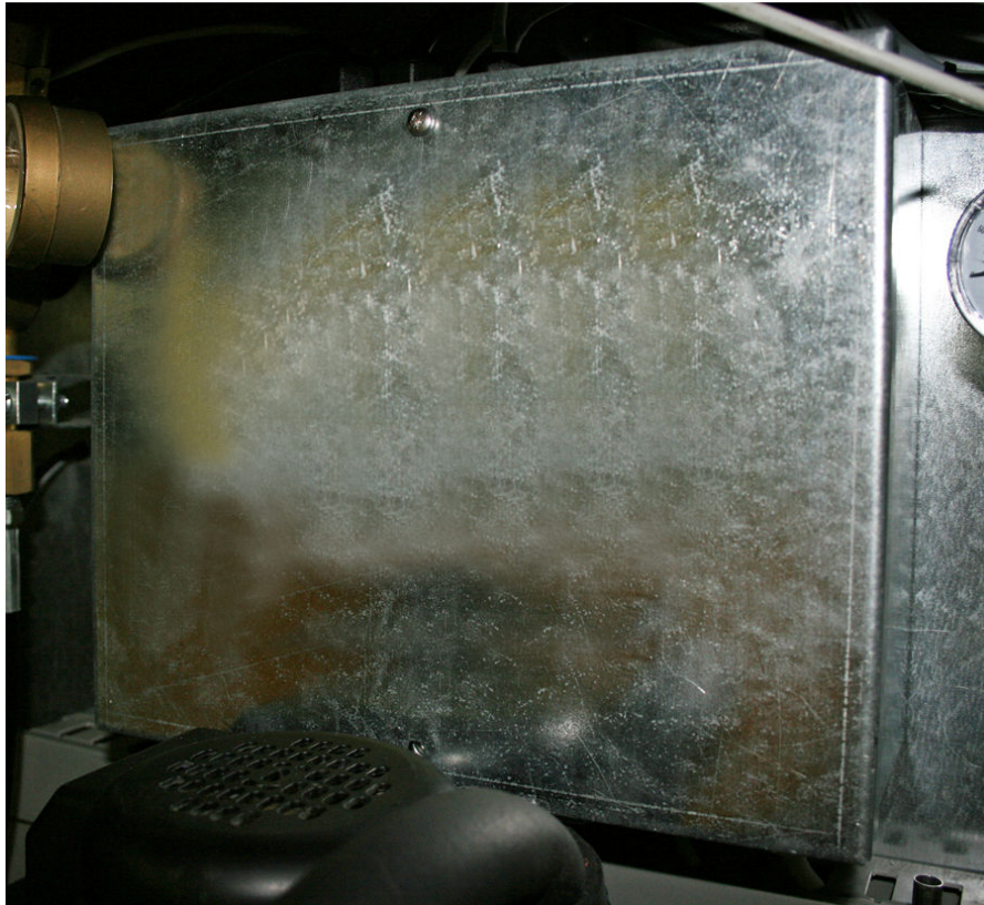
Figure 9 - Internal control box
