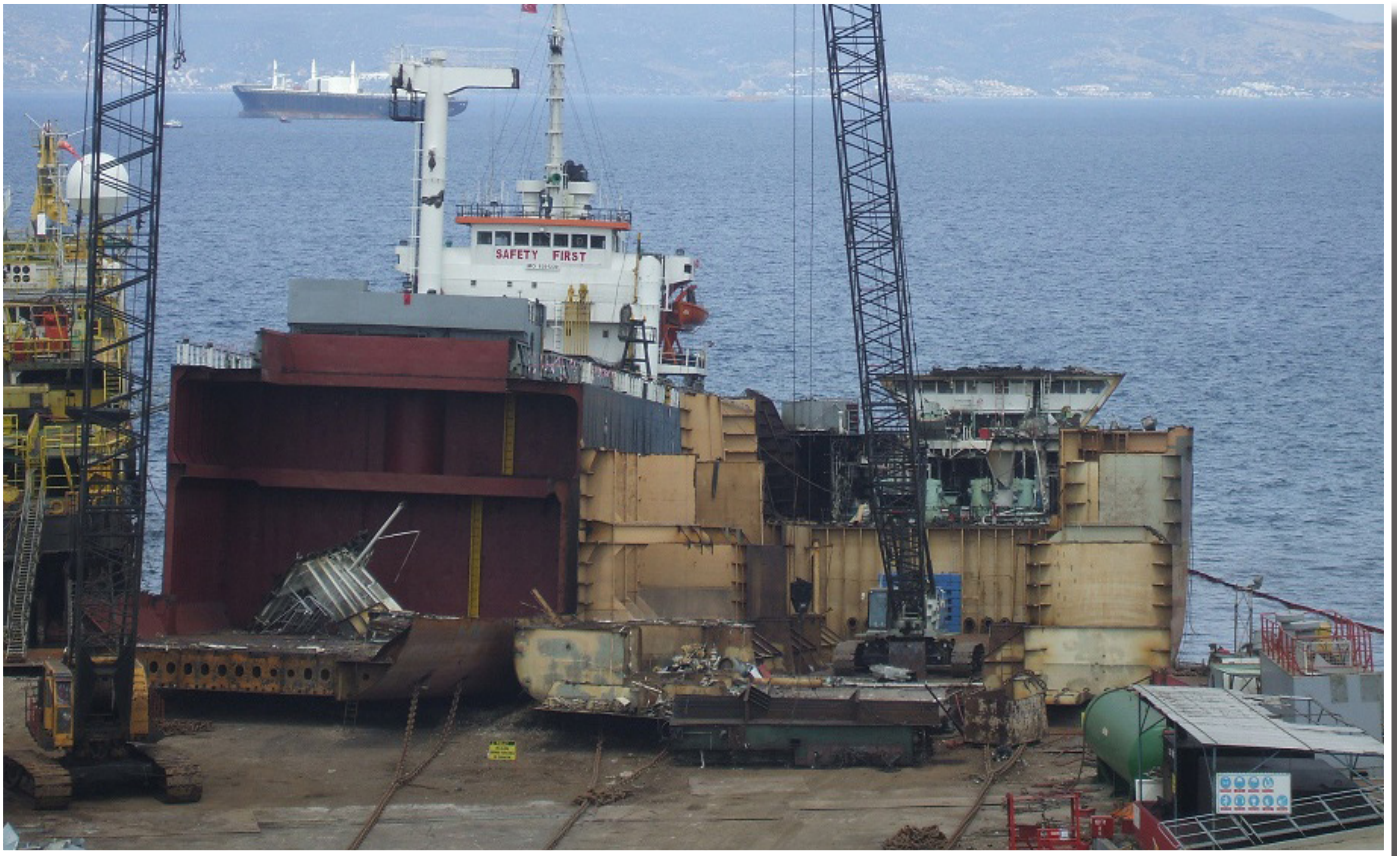
10 May 2016 The ship is now on the slipway where materials are segregated and processed.
