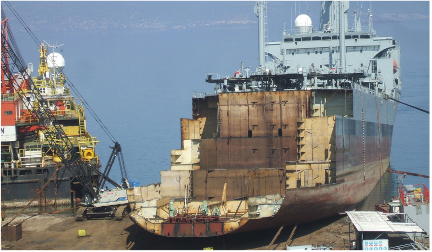
31 March 2016 The ship is now on the slipway. The vessels superstructure is dismantled while the vessel is afloat reducing its weight.
