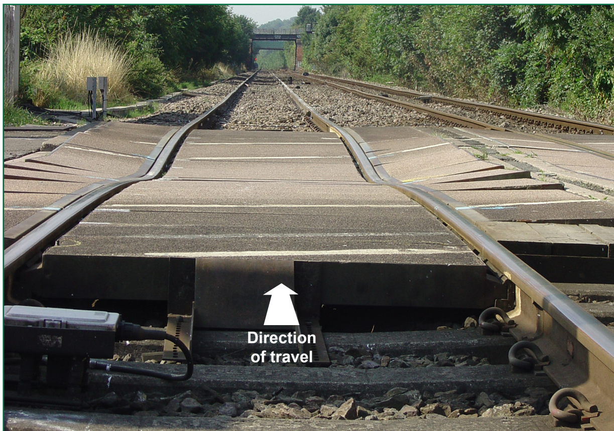
Figure 3: The dip in the rails at the point of derailment
