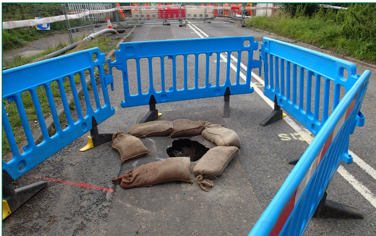
Figure 8: Hole in the road found on 8 August 2013 (photograph taken on day of accident)
