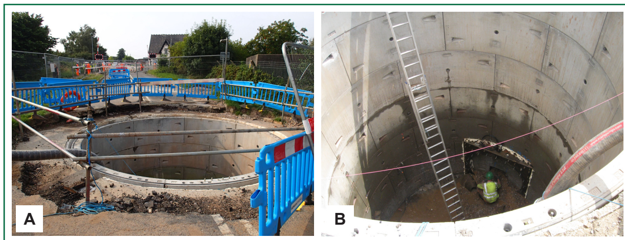
Figure 6: Launch shaft (a) and reception shaft (b) during the works (image courtesy of Morgan Sindall)
