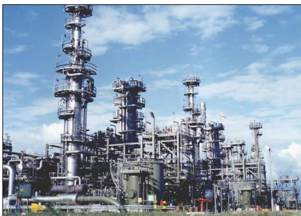
Photo 5 - POA Gas Terminal Process Train
