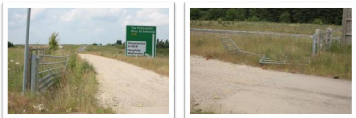
Figure 5-27 – Damaged access gate on the bridleway at the western end of the environmental barrier near Stowmarket.
