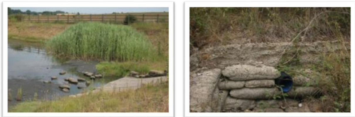
Figure 5-22 – Detached sandbags in the balancing pond opposite Gallows Field (left), and missing sandbags at the Tot Hill culvert/ Balancing Pond 3 (right).
