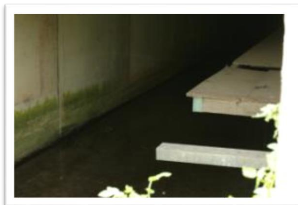
Figure 5-20 – The broken mammal ledge at Tot Hill culvert (north).
