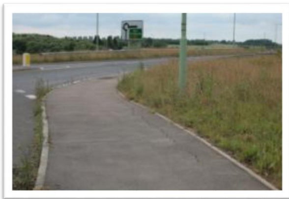
Figure 5-24 – Section of cracking along the northern NMU approach to the new Tot Hill overbridge
