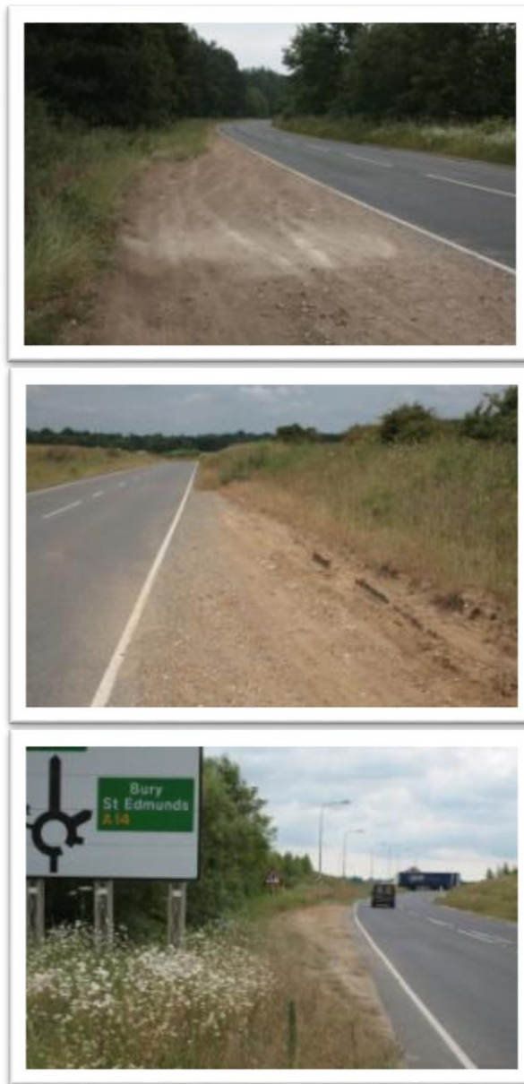
Figure 5-13 – Bare and rutted areas of verge along the eastbound carriageway of the old A14/ local access road; just east of Haughley New Street (upper), directly west of Fishponds Way (centre), and on the approach to Tot Hill junction (lower).
