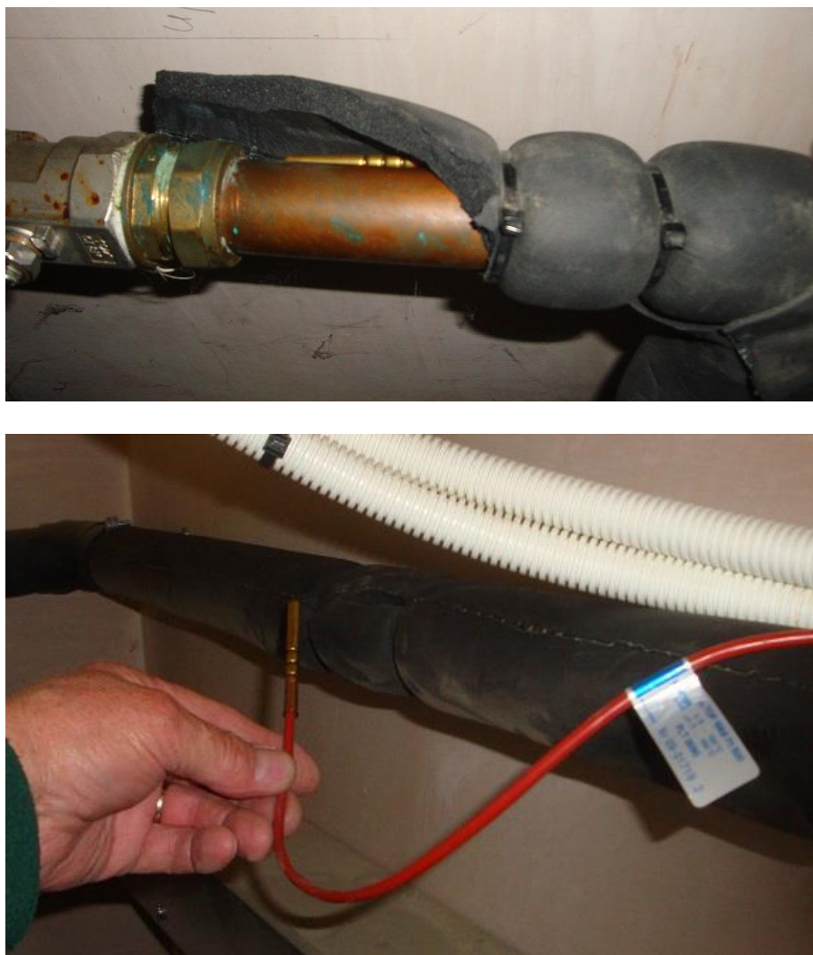
Figure 65 – Loose temperature sensors on the wrong pipes
