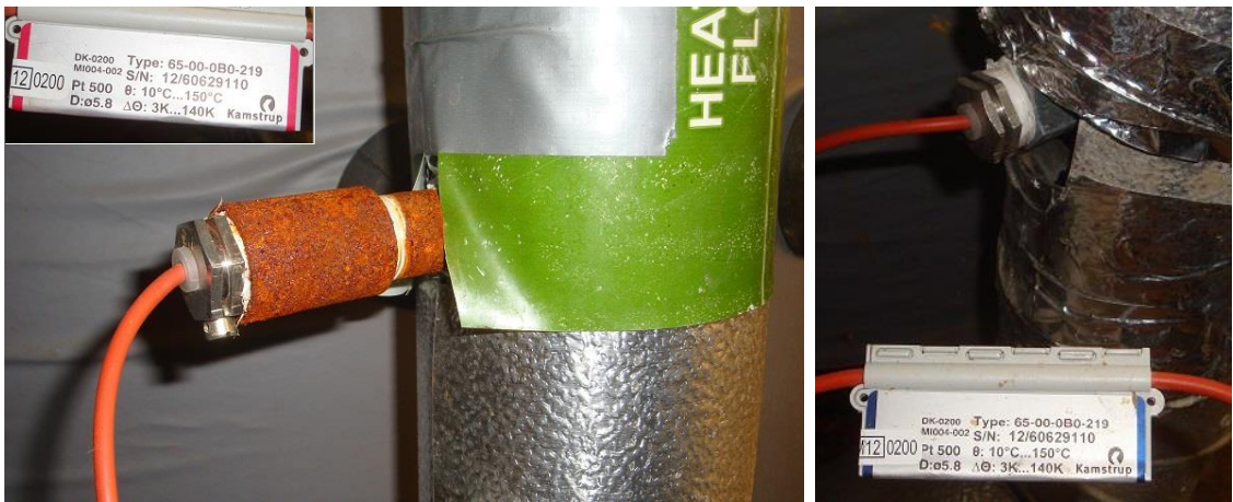
Figure 63 – A made-up fitting and a correct fitting used on the same heat meter.
