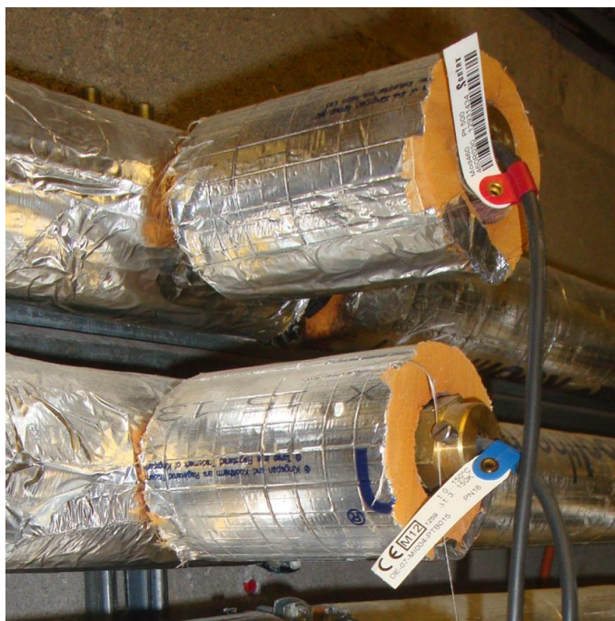
Figure 62 – Incorrectly designed sensor fittings
