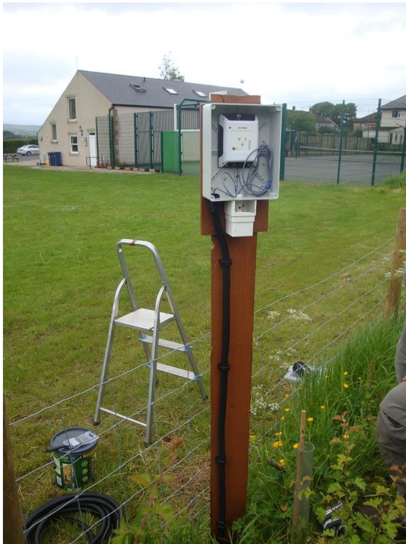
Figure B 14 – Outdoor ground and air temperature measurement assembly.
