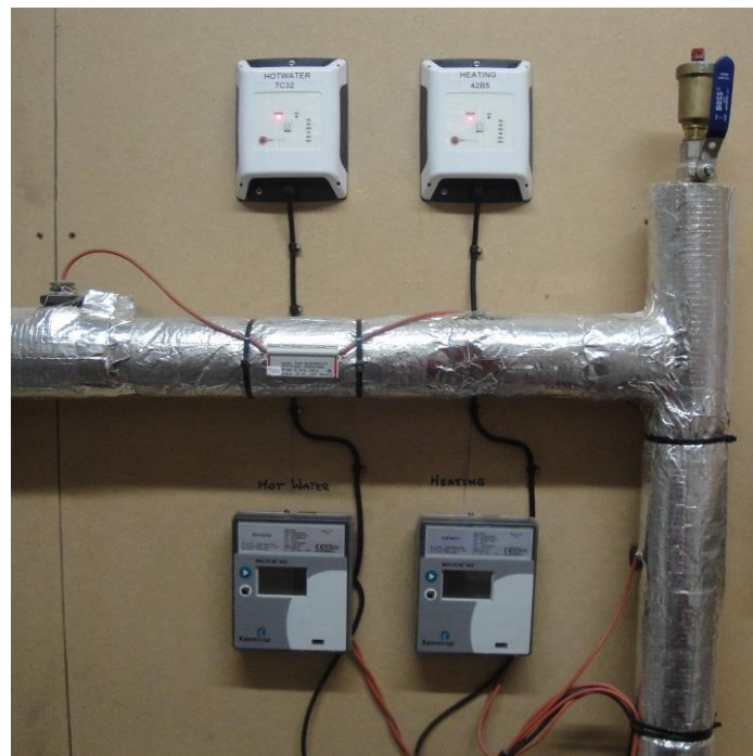
Figure B 16 – ZPC-10 pulse counters connected to battery-powered heat meters
