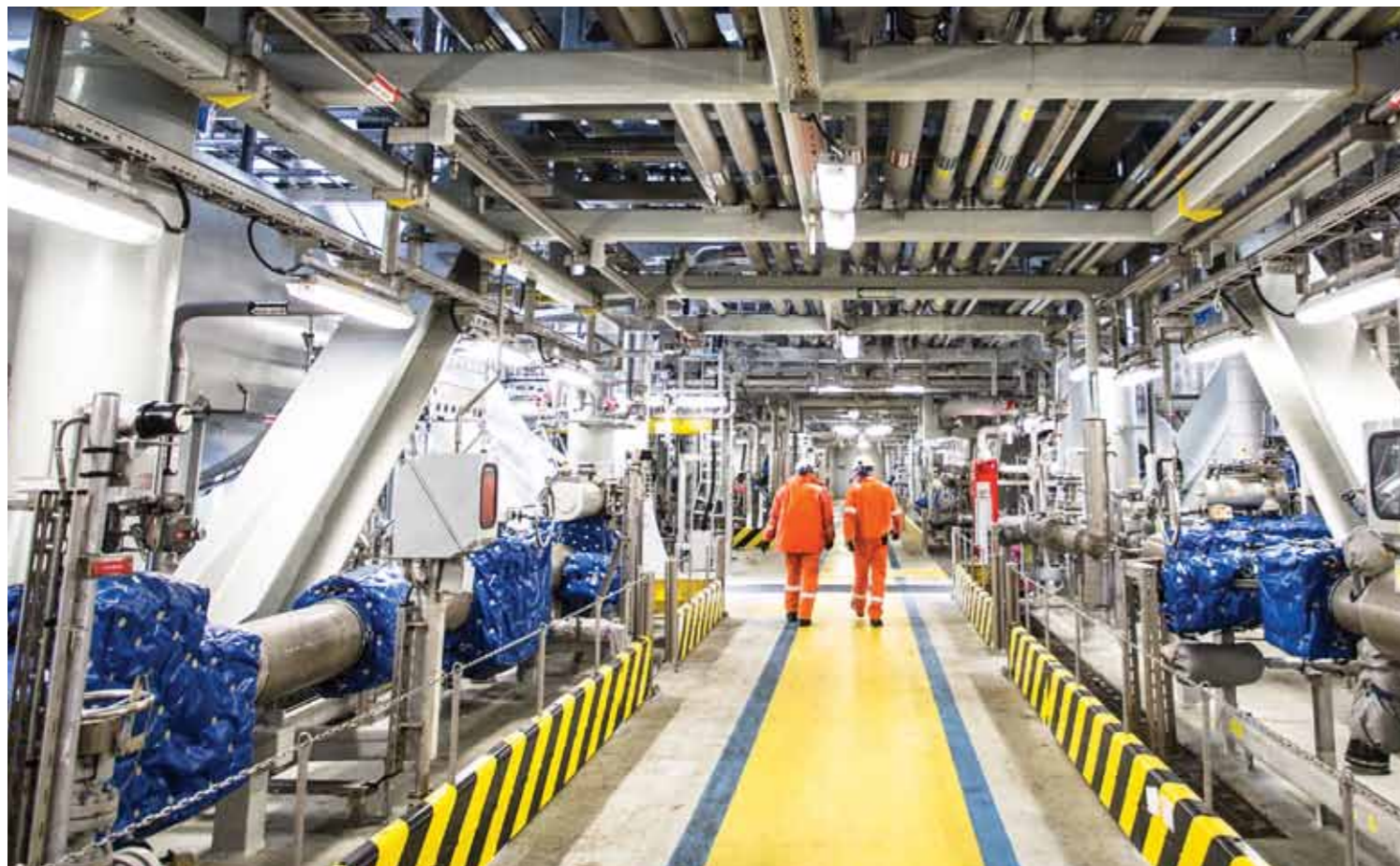
► Skarv FPSO walkway
