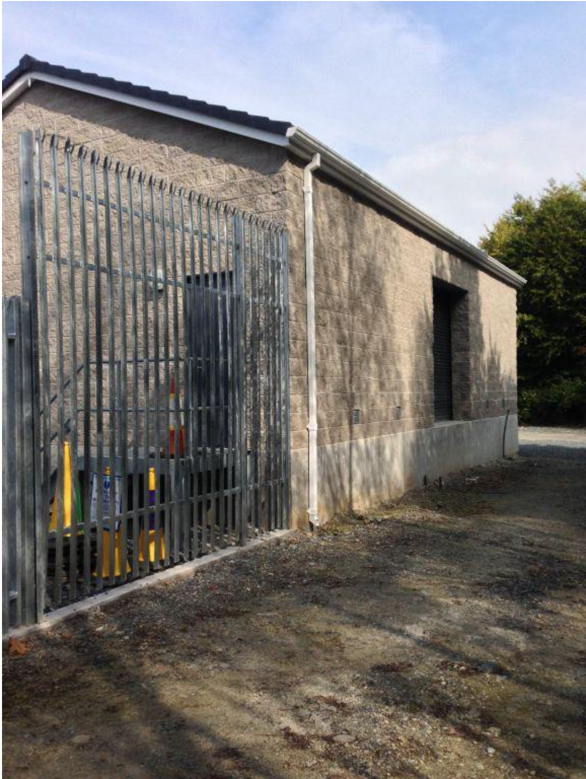
High voltage switch room under construction on a raised plinth. (Courtesy NIE)
