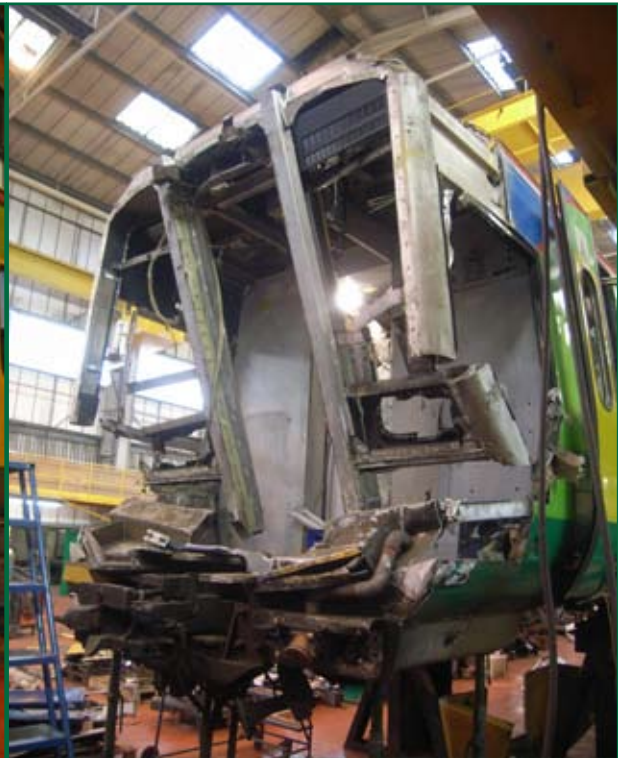
Figure 6: Damage to superstructure (fairings and flexible gangway removed)
