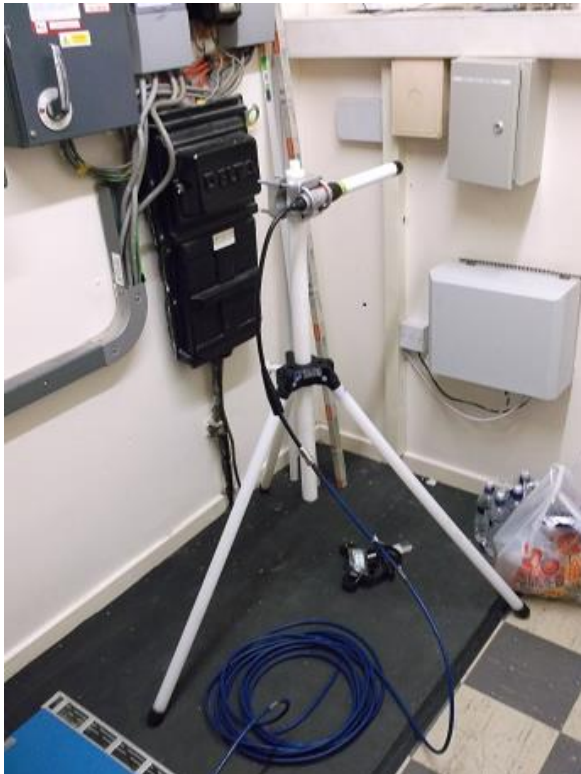
Figure 4 Transmit Location 1 Electricity Cupboard
