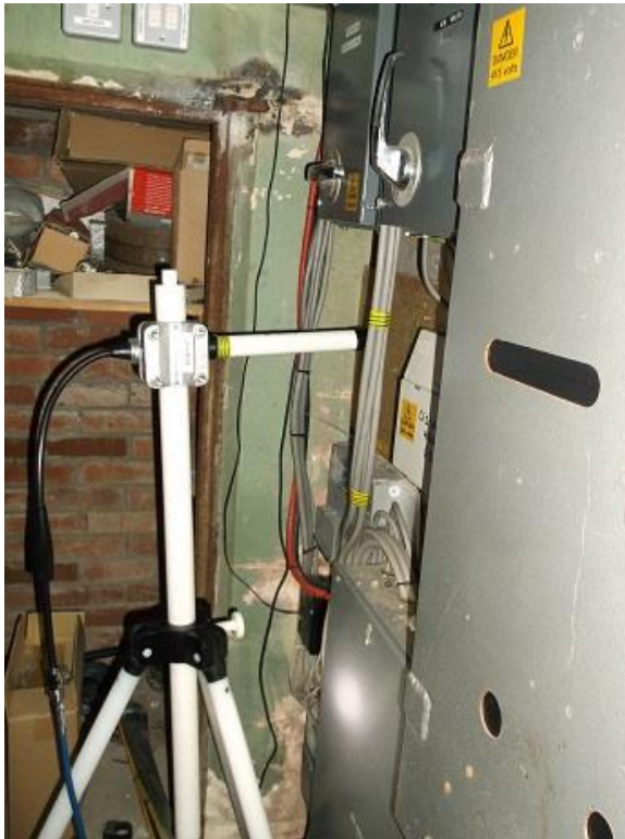
Figure 4 Transmit Location 1 Electricity Cupboard (Room 49)
