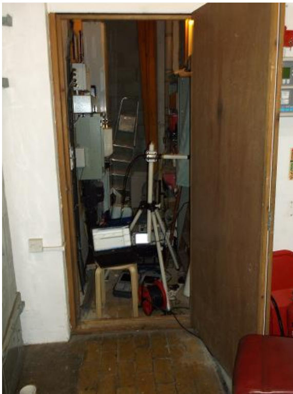
Figure 4 Transmit Location 1 Electricity Cupboard
