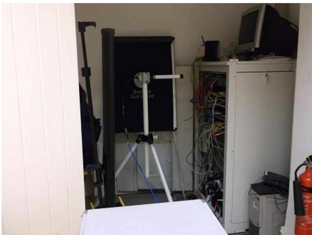
Figure 6 Transmit Location 3 IT Office (Room 88)
