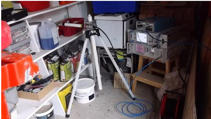
Figure 3 Transmit Location 1 Electricity Cupboard
