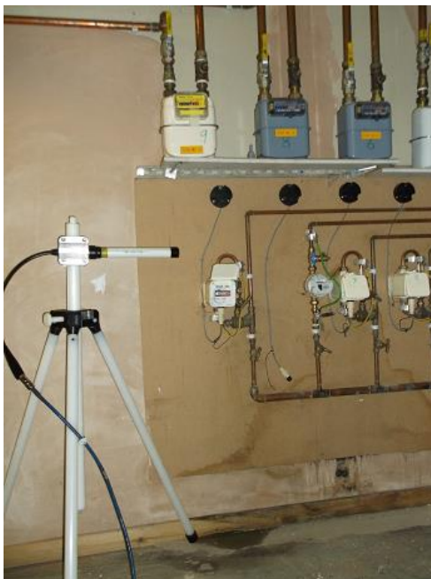
Figure 3 Transmit Location 1 Electricity Cupboard
