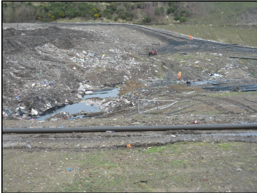
Ponding leachate in centre of cell 3 – in January (prior to remedial works)
