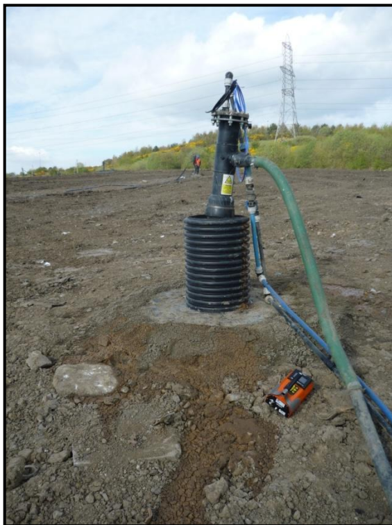
Sealed gas extraction well (within cell 3)
