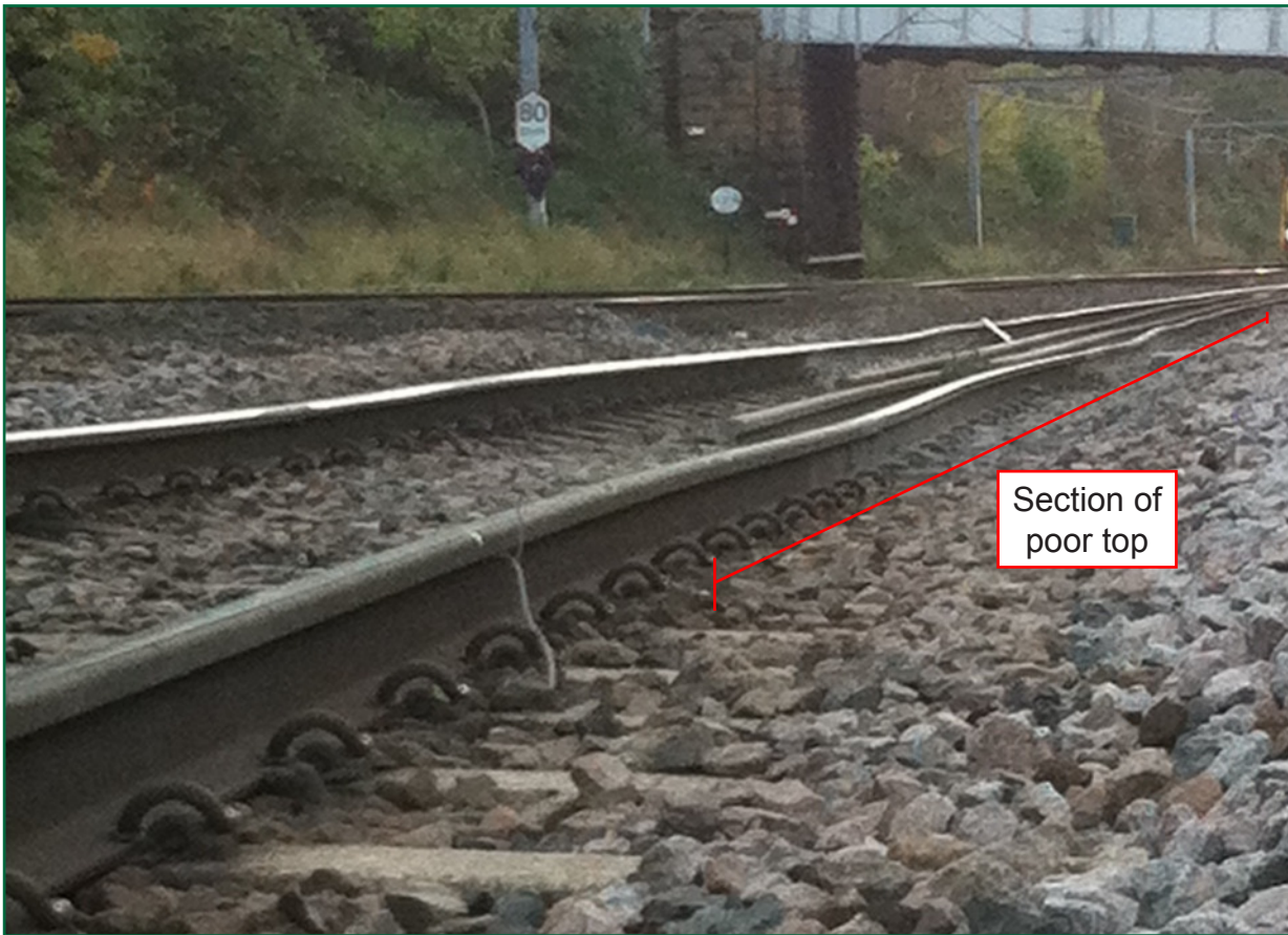
Figure 20: The variation in the height of the rails on the approach to the point of derailment (image courtesy of Network Rail)
