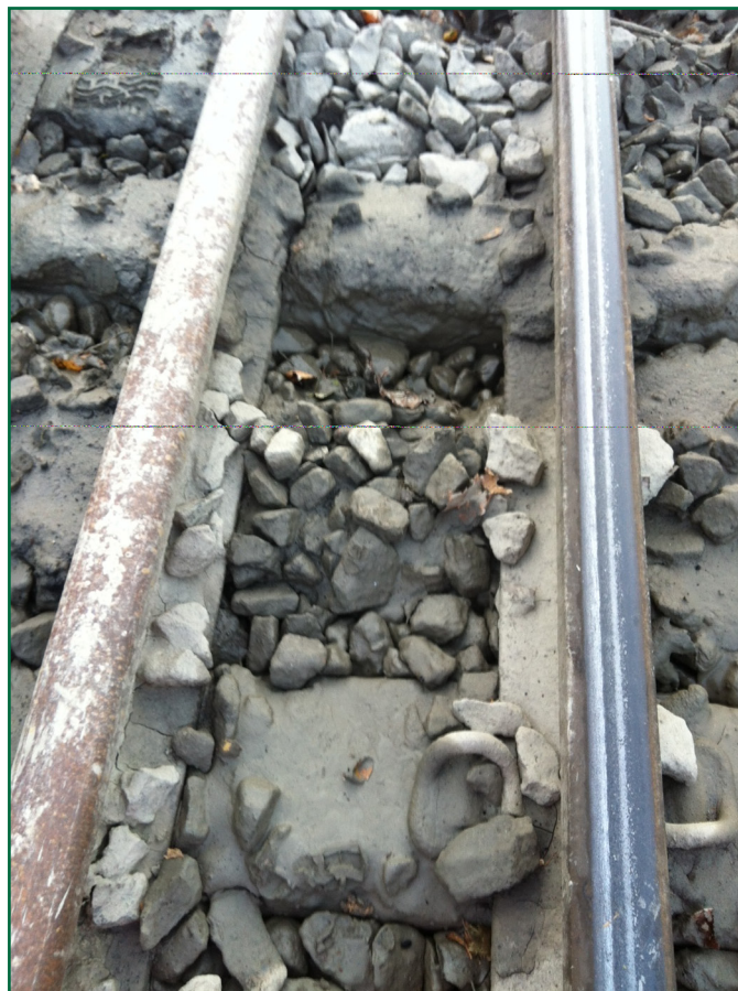
Figure 24: Close up view of a wet bed at the point of derailment on the Down Sunderland line (image courtesy of Network Rail)
