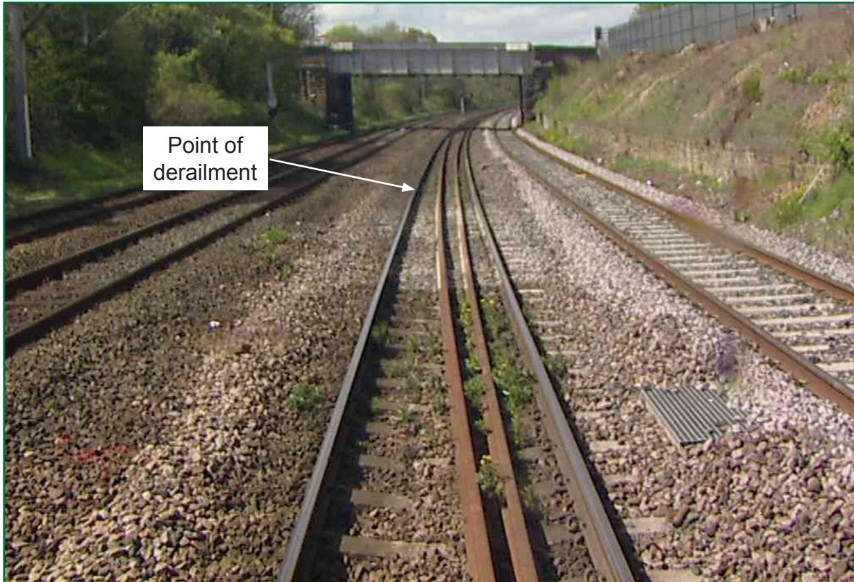
Figure 23: Footage recorded in May 2014 showing vegetation growing in the four foot of the Down Sunderland line (image courtesy of Network Rail)
