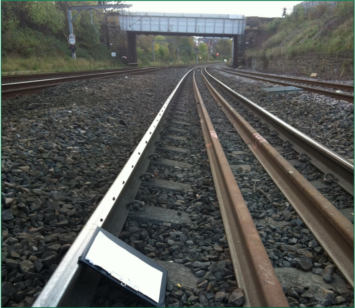
Figure 5: The path of the flange marked out on the head of the left-hand rail (image courtesy of Network Rail)
