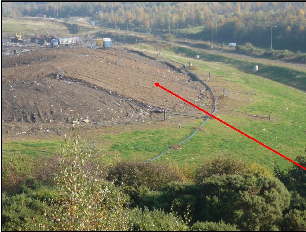
Cohesive sealing layer being progressively applied in advance of further capping works
