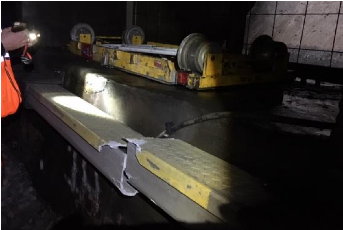
Undamaged trolley as found within the pressure relief shaft No. 1 recess in Stowe Hill Tunnel. The metal grille at the bottom of the shaft can be seen in the background (photo courtesy Network Rail)
