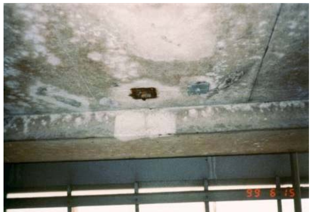
Corrosion of galvanised holding down bolts
