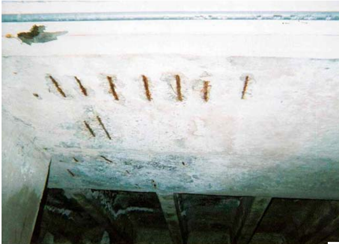
Photograph 4 Example of sagging reinforcement, low cover & corrosion spalling
