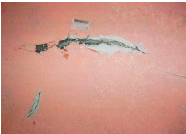
Photograph 8 Typical example of premature deterioration of a waterproof membrane due to defective installation & inadequate crack bridging capability
