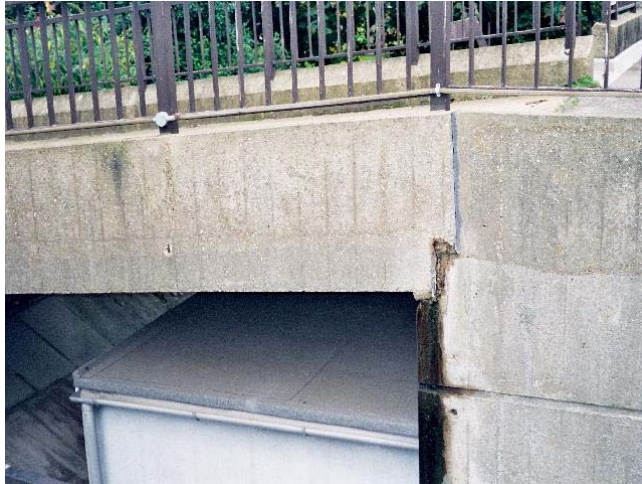
Photograph 15 Typical example of a seeping half-joint
