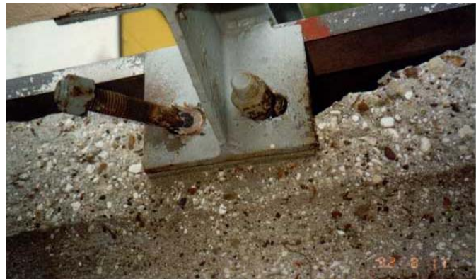
Photograph 10 Typical example of chloride-induced corrosion of fixing bolts for cladding.
