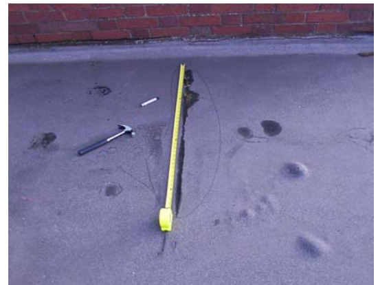
Blistering and failure of waterproofing membrane
