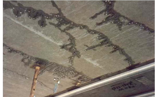
Typical example of leakage through shrinkage cracks in reinforced concrete deck slab
