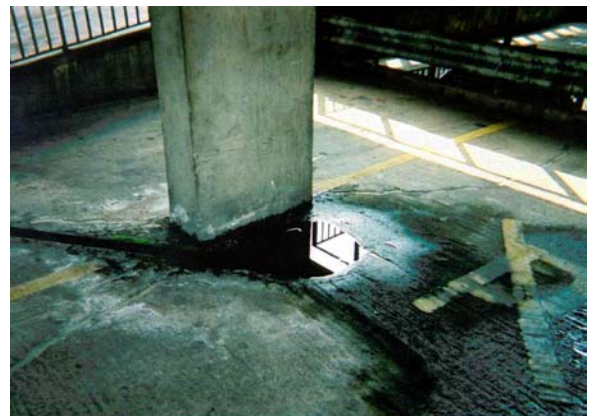
Example of water ponding around the base of a column due to ineffective gully outlet.
