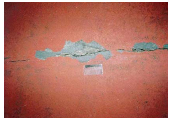
Typical example of failed membrane caused by its inability to bridge existing cracks in the underlying concrete.
