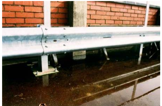
Ponding of water around base plates and holding down bolts.
