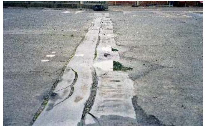
Failed joint with water ponding
