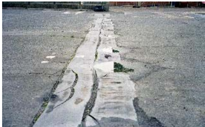
Photograph 7 Typical example of poorly constructed movement joint suffering premature deterioration
