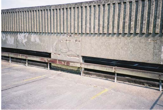
Photograph 11 Typical example of carbonation-induced corrosion of reinforced concrete
