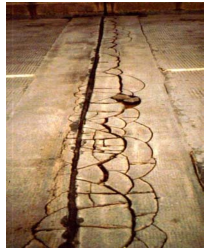
Degraded joint area
