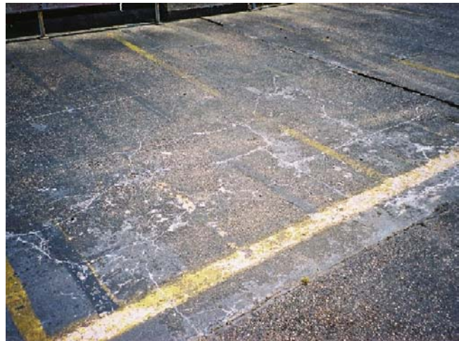
Photograph 12 Typical example of frost damaged deck slab on unsurfaced car park roof
