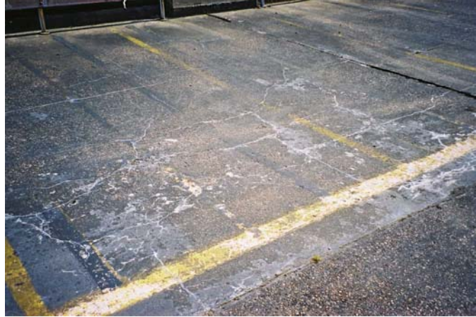
Photograph 2 Typical example of combined erosion/abrasion and frost damage of a concrete deck.
