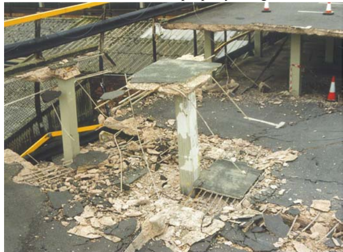
Photograph 16 Example of column head shear failure at Piper's Row
