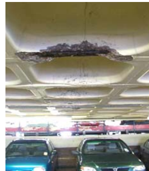
Large sections of soffit have spalled away due to rusting of the reinforcement beneath.
