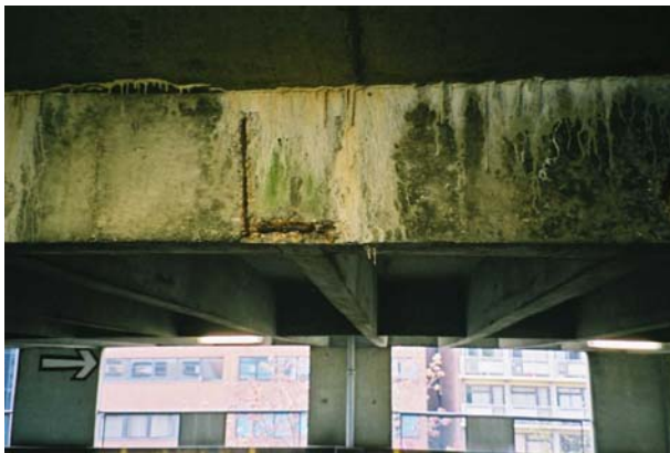
Photograph 6 Typical example of poorly placed reinforcement leading to low cover and corrosion spalling
