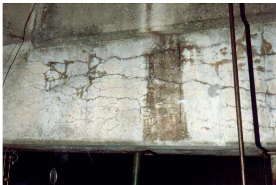
Typical example of ASR-related cracking & damage.
