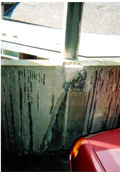
Similar defects occur when poorly cast fixing pockets for external cladding (such as pre-cast concrete mullions) crack and spall.
