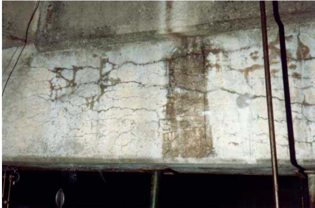
Photograph 13 Typical example of ASR damage of a reinforced concrete beam
