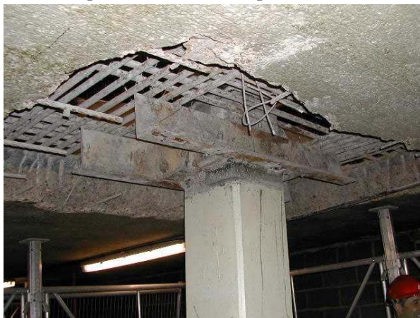
Photograph 14 ‘Opening-up’ of column in a lift slab structure where bottom reinforcement does not extend to the lifting collar, nor is it properly anchored
