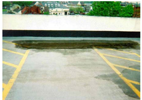
Water ponding on roof due to incorrectly fitted drainage gully
