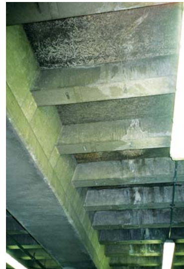
Water leakage from failed joint as viewed from the underlying soffit.
