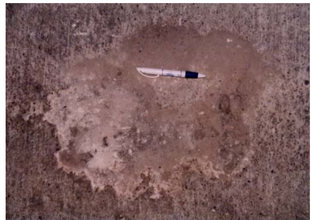
Surface damage to concrete driving aisle (Picture courtesy of BRE Limited)
