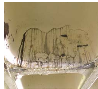
Rust staining resulting from corroding reinforcement caused by carbonation of concrete combined with the ingress of water.
