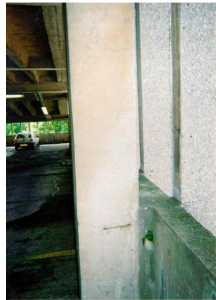
Corrosion of reinforcement & cracking
