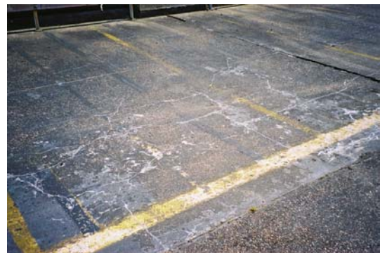
Typical example of freeze-thaw damage & cracking.
