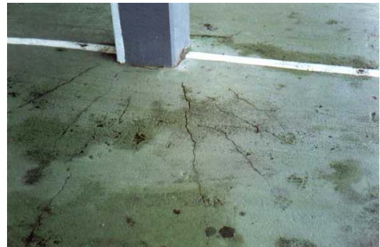
Typical example of radial cracking from around a column associated with flat slab.
