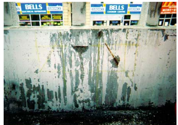
Corroded reinforcement exposed by spalling of the internal face of a parapet.
