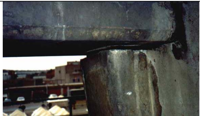
Photograph 19 Typical example of joint seepage & corrosion on a bearing shelf
