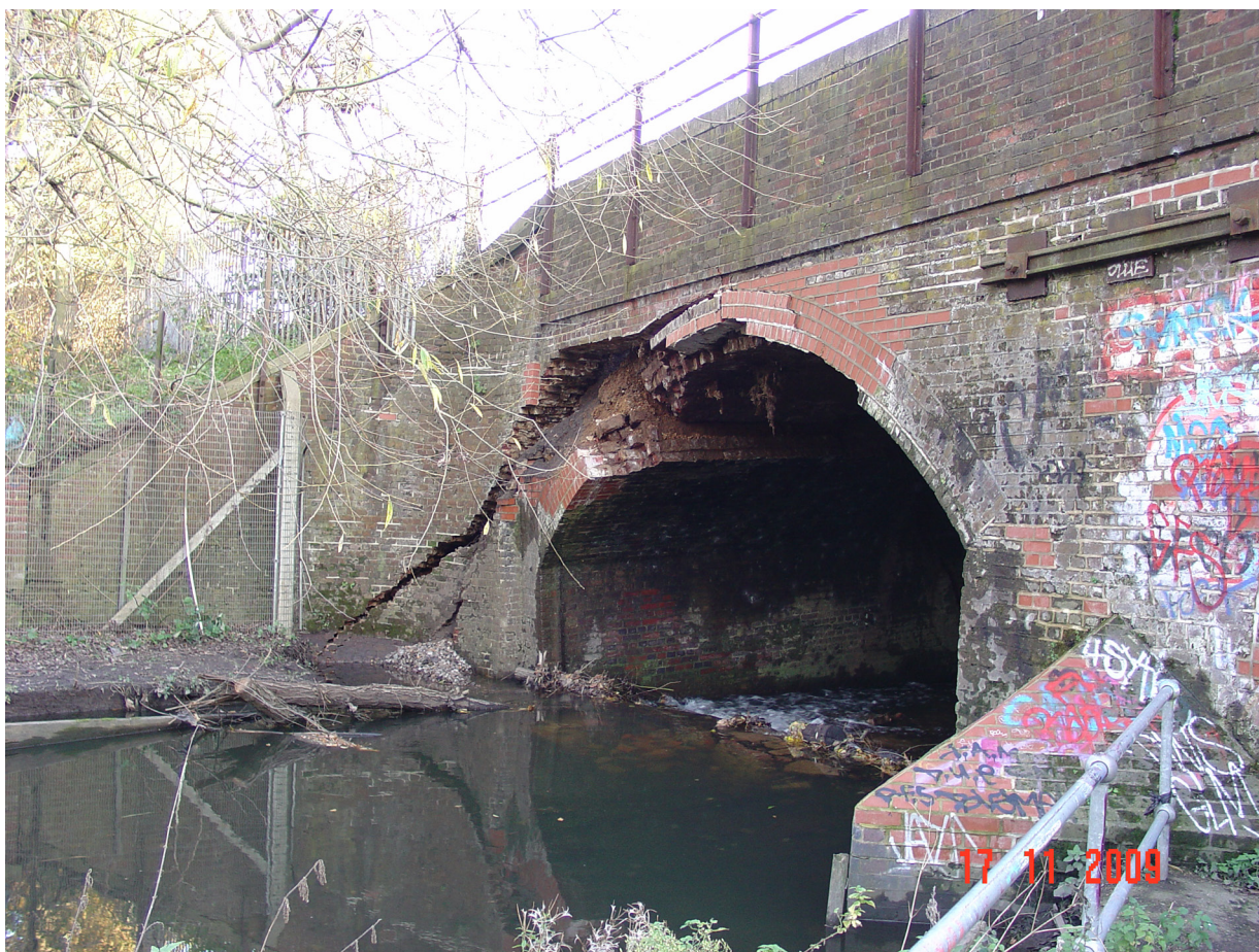
Figure 22: Bridge RDG1 48, spanning the River Crane between Whitton and Feltham in west London. The arch failed after its abutment was undermined by scour erosion on 15 November 2009.
