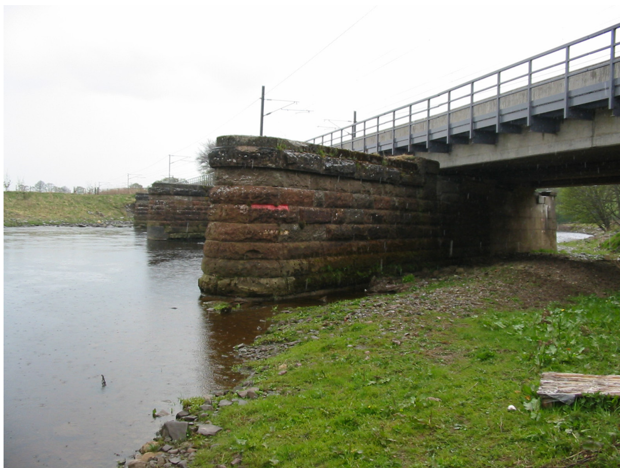
Figure 20: Red marker visible on upstream end of pier 1 in 2003 (photograph courtesy of Network Rail)
