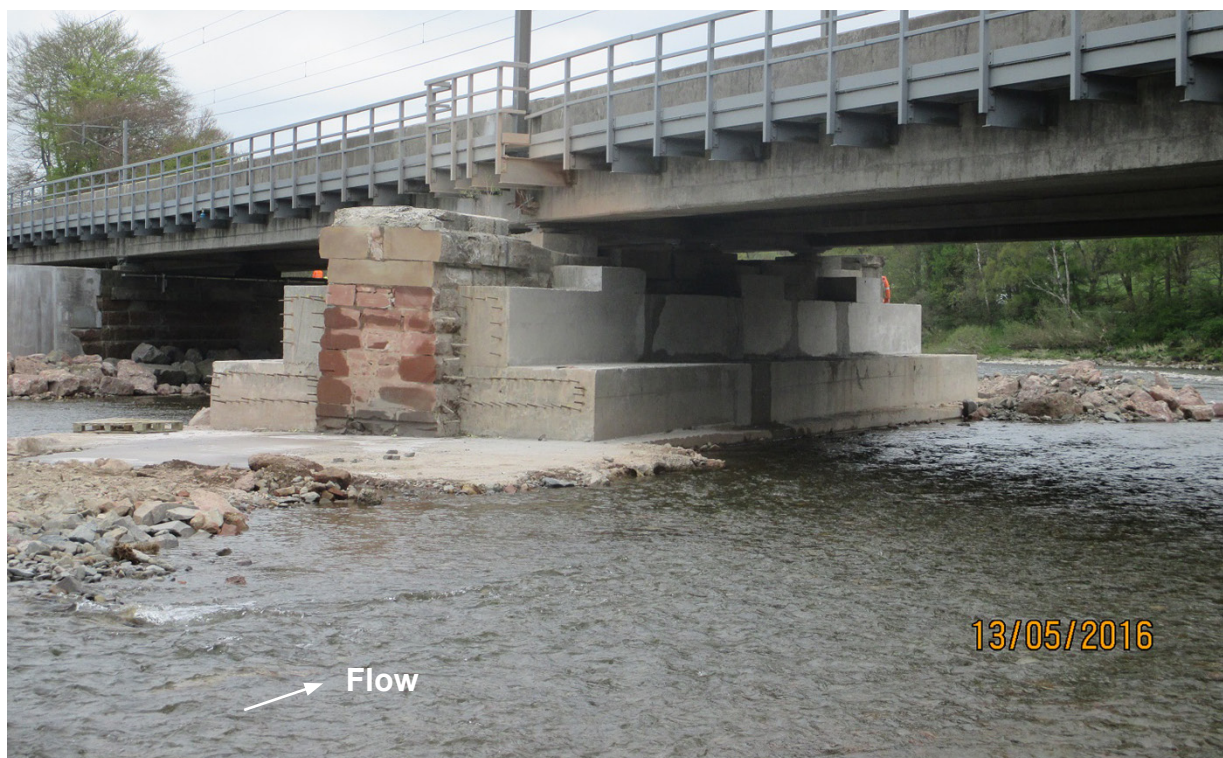
Figure 16: Pier 2 stabilisation works after removal of upstream end (photograph courtesy of Network Rail)
