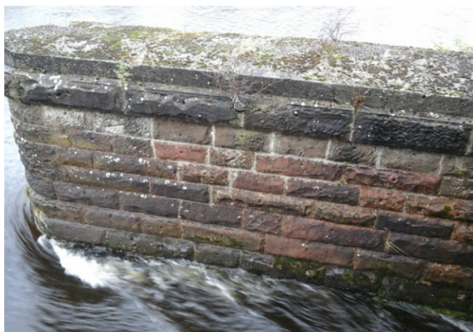
Figure 21: Upstream end of pier 2 on 9 December 2015, seen during a visual examination three weeks prior to the incident (photograph courtesy of Network Rail)
