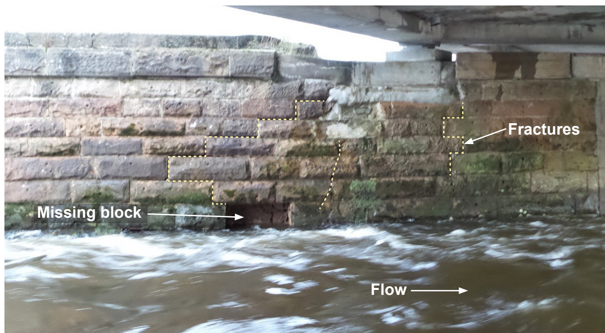
Figure 9: South face of pier 2 on 31 December 2015 showing missing block and fractures (photograph courtesy of Network Rail)
