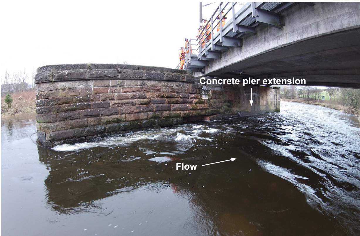
Figure 11: South face of pier 2 on 1 January 2016 prior to start of emergency stabilisation works. Note that the operative's safety harness is anchored to the adjacent overhead electrification mast (photograph courtesy of Network Rail Air Operations).
