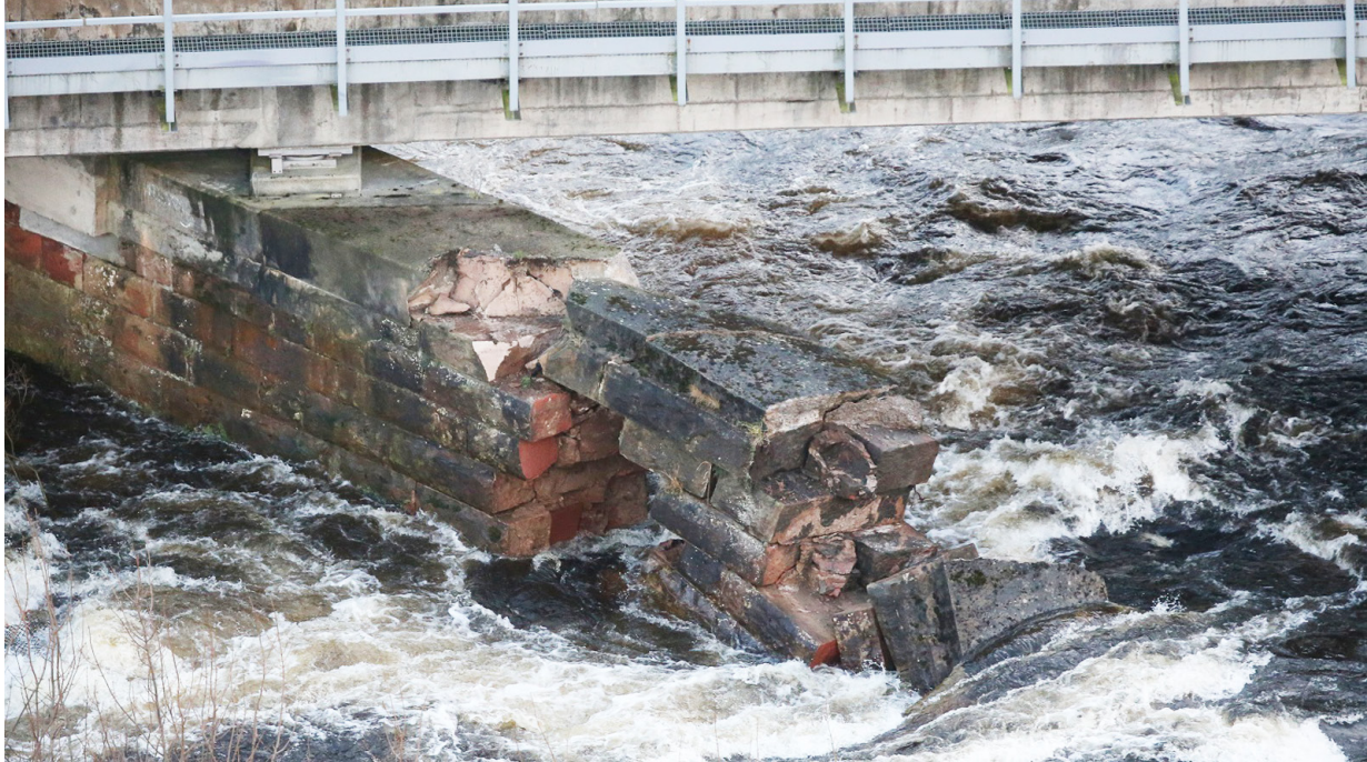
Figure 14: Scour damage to redundant section of pier 3 on 10 January 2016 (photograph courtesy of Network Rail Air Operations)
