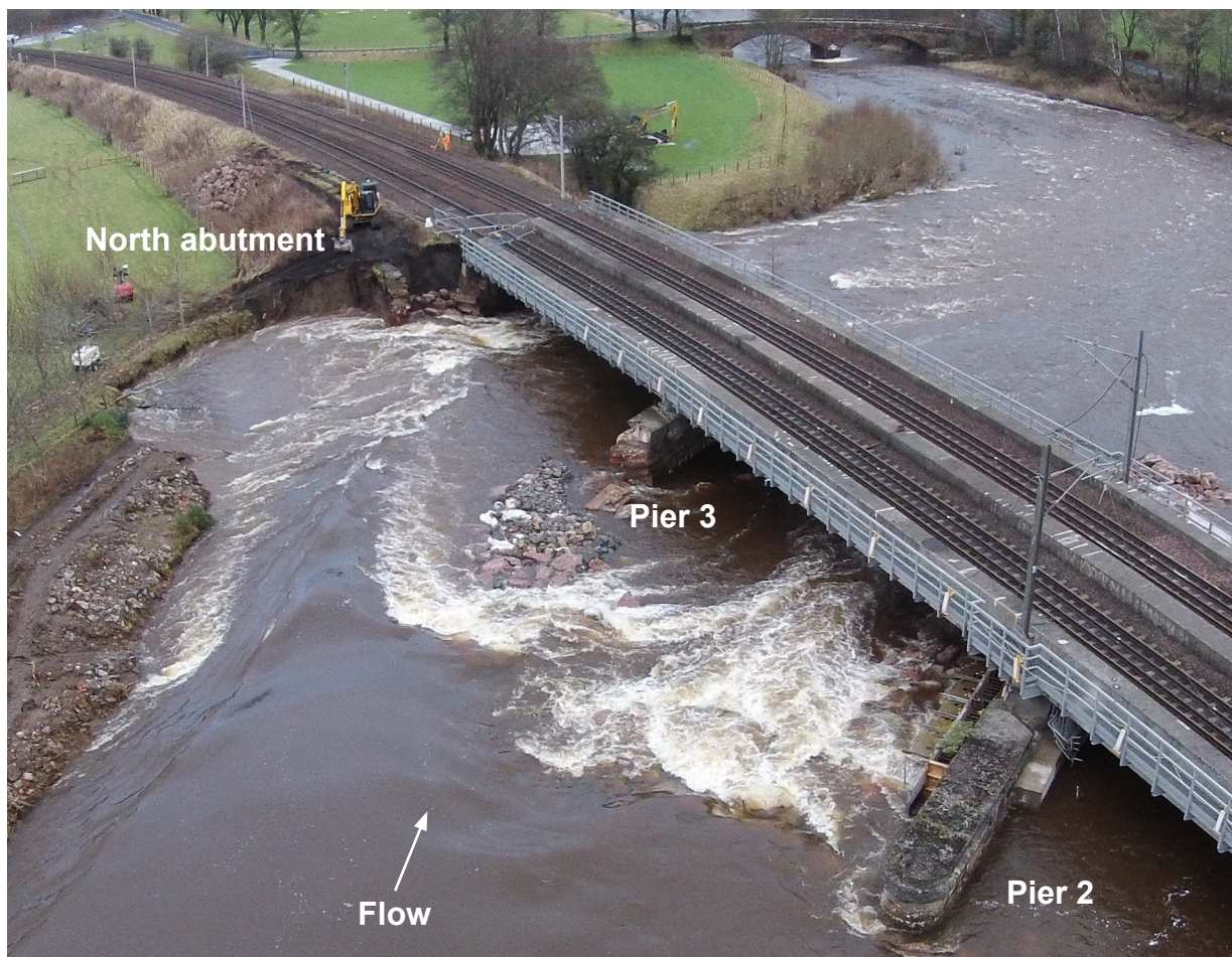
Figure 15: Scour damage to north abutment and embankment on 27 January (photograph courtesy of Network Rail Air Operations)
