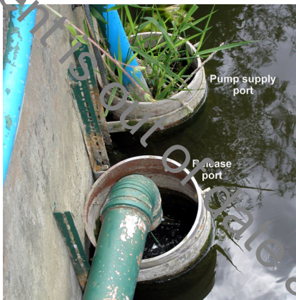
Figure 4.2.6 Water supply and release ports for Strensham right-bank eel pass
