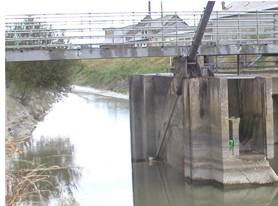
Figure 4.3.11. Plancoet Dam from upstream. The sluice is open so the water surface is well below the usual retained level.
