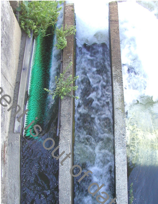
Figure 4.3.19. Detail of eel pass at Moulin a Pigné
