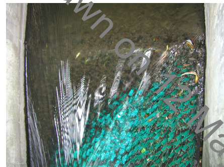
Figure 4.2.20. Staines Lino Mill Weir – top of bristle ramp. Note fast flow and erosion of bristles.
