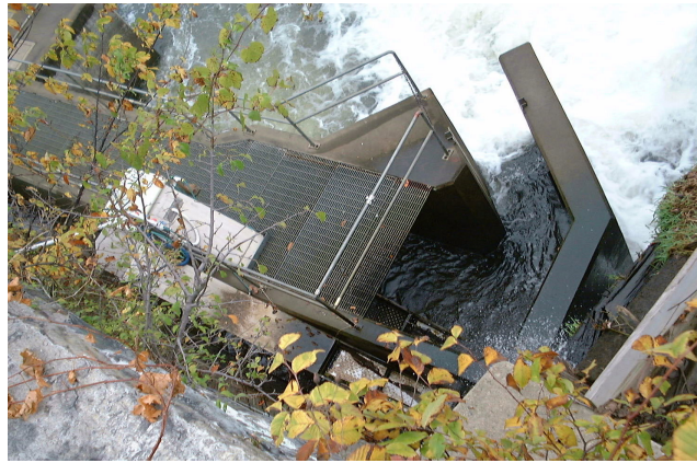
Figure 4.4.15. Eel pass-trap at Westfield Dam viewed from above. The eel pass is the pale grey installation on top of the Denil fish pass. The eel pass has two ramps, one collecting fish from within the fish pass, the other from between the fish pass and the dam wall.
