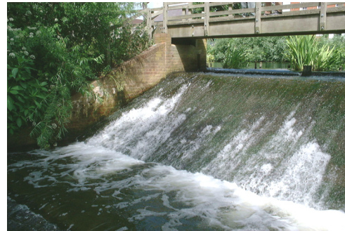
Figure 4.2.16. Cobham Mill Weir. Note vertical lip at weir crest, and broken water due to roughened surface.
