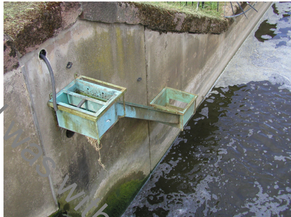
Figure 4.2.4 Left bank elver pass at Stanchard Pit, with lower ramp missing due to flood damage.
