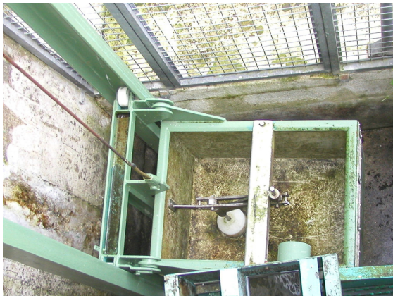
Figure 4.3.14. Lift hopper at Ville Hatte Dam eel pass in lower level position.
