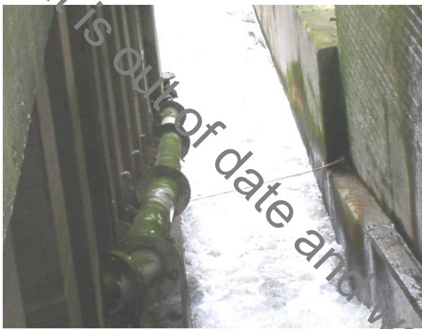
Figure 4.2.21. View down the fish pass at Barking Barrage at low tide. The elver pipe pass is on the left, and passes through the wall of the fish pass. The top of the perforated vertical stand pipe that represents the entrance of the pipe pass is just visible at the far end.
