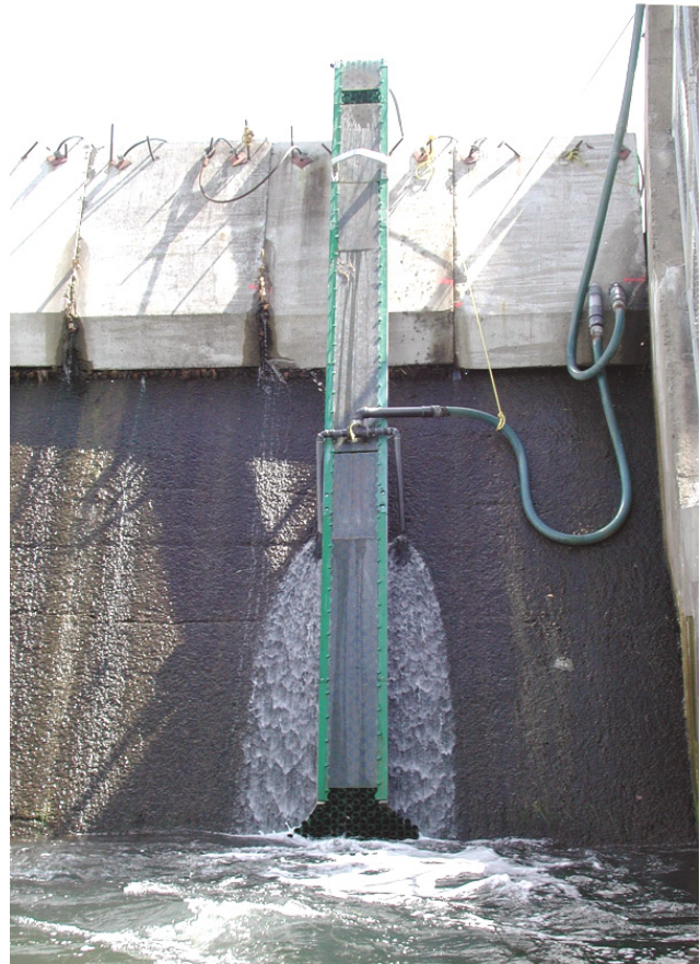
Figure 4.4.3. Eel pass at Chambly Dam. Note the breakwater blocks on the dam crest, and the gravity-fed attraction water being discharged from two pipes part way down the dam face. Photo D. Desrochers
