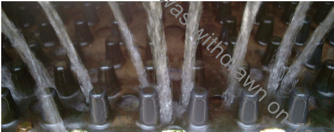
Figure 4.4.16 Top of one of the ramps at the Westfield pass-trap showing the Akwadrain substrate and the jets of water irrigating the ramp.
