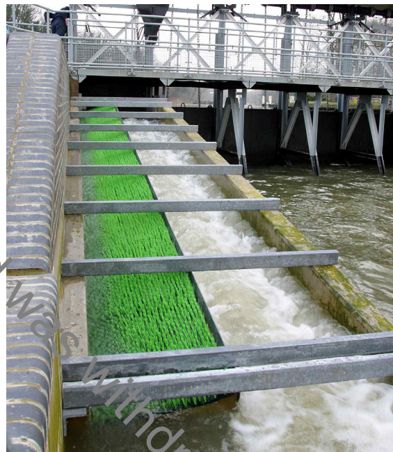
Figure 4.2.13 Abingdon Weir eel and baffle passes, covers removed, Feb 2003
