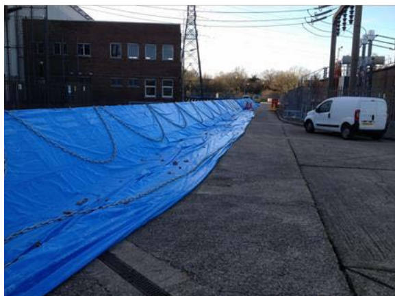
Temporary flood barrier deployed at Watford South Switching Station (February 2014)
