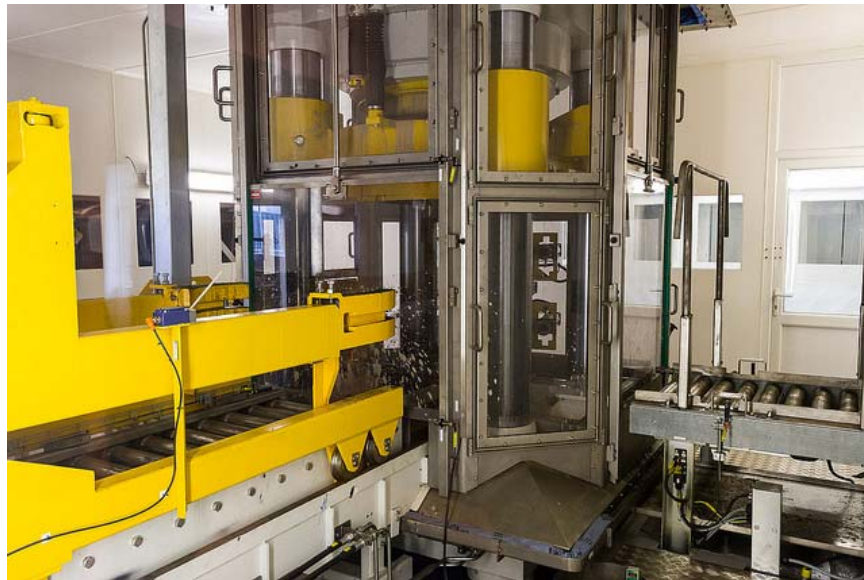
Figure 37: The supercompactor at Dounreay
