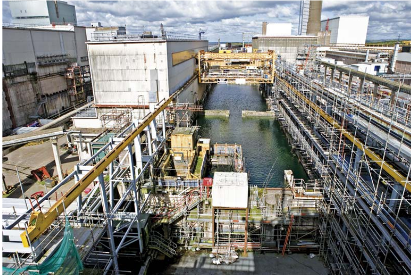
Figure 32: First Generation Magnox Storage Pond (FGMSF) at Sellafield
