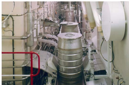
Figure 27: Encapsulation line at Sellafield Waste Packaging and Encapsulation Plant (WPEP)
