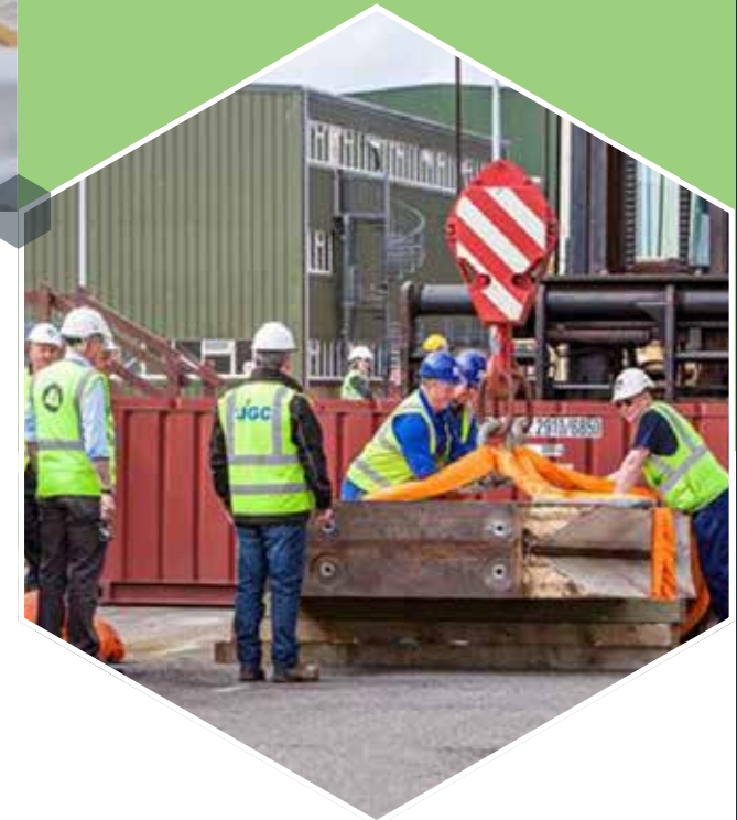
Photographs: Above, a section of wall ready for lifting and (inset) one of the 26-tonne doors ready for transfer to the LLW facility after being winched out through the roof
