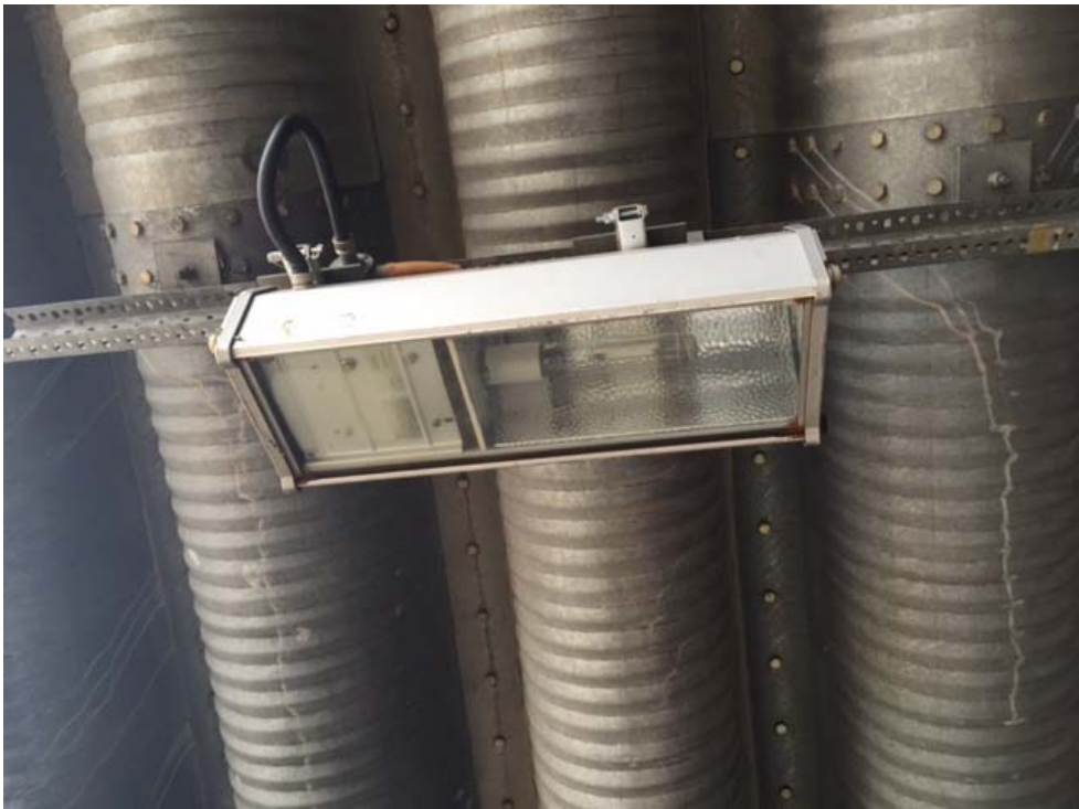
External View of Installed Fitting
