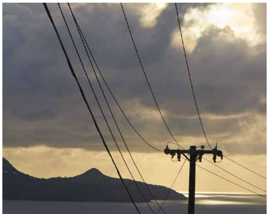
Power line on Mayreau Island, St Vincent and the Grenadines
