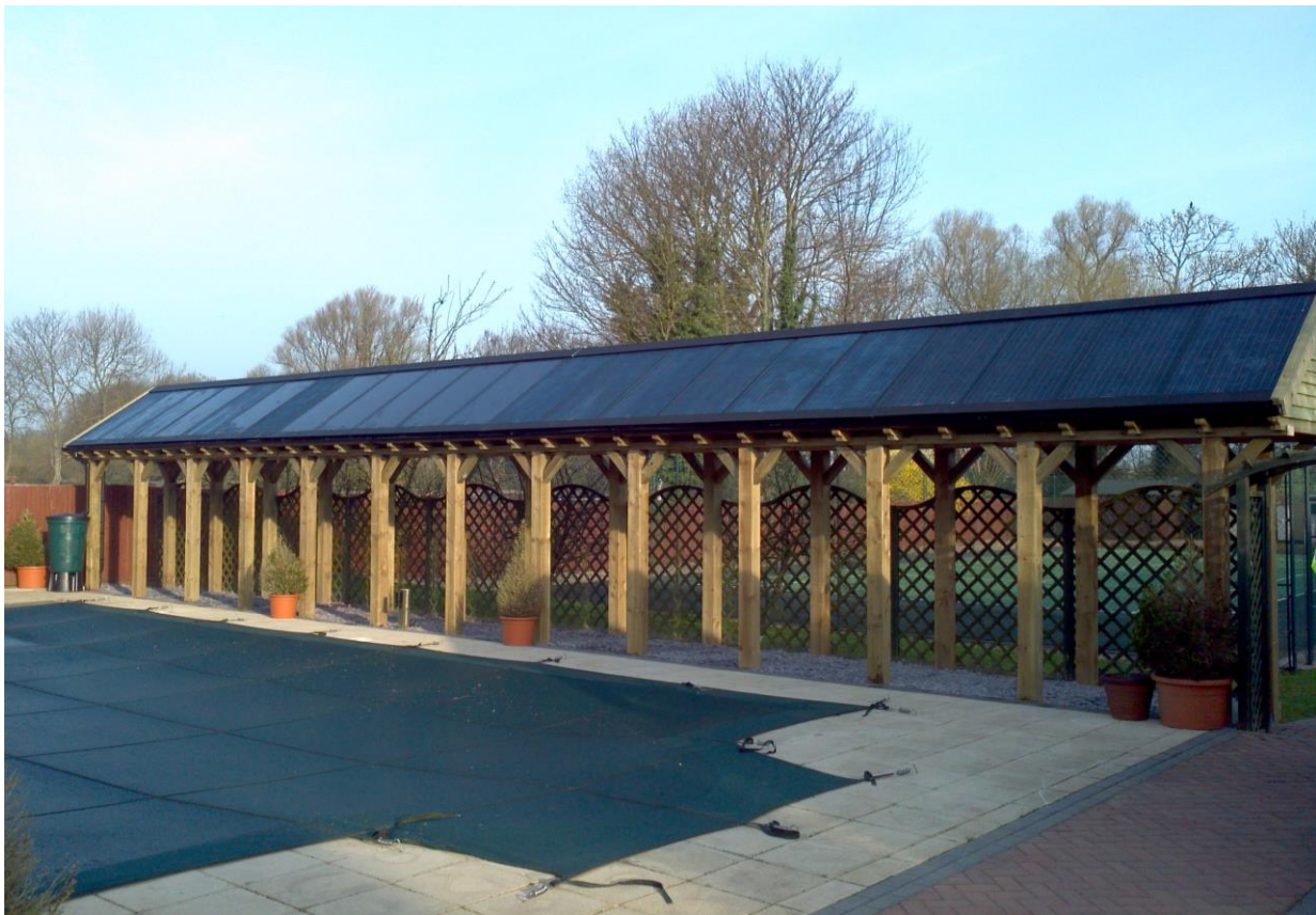
Figure 17 Installation of PV-T to provide heat for a swimming pool. Image courtesy of Anthony Morgan.
