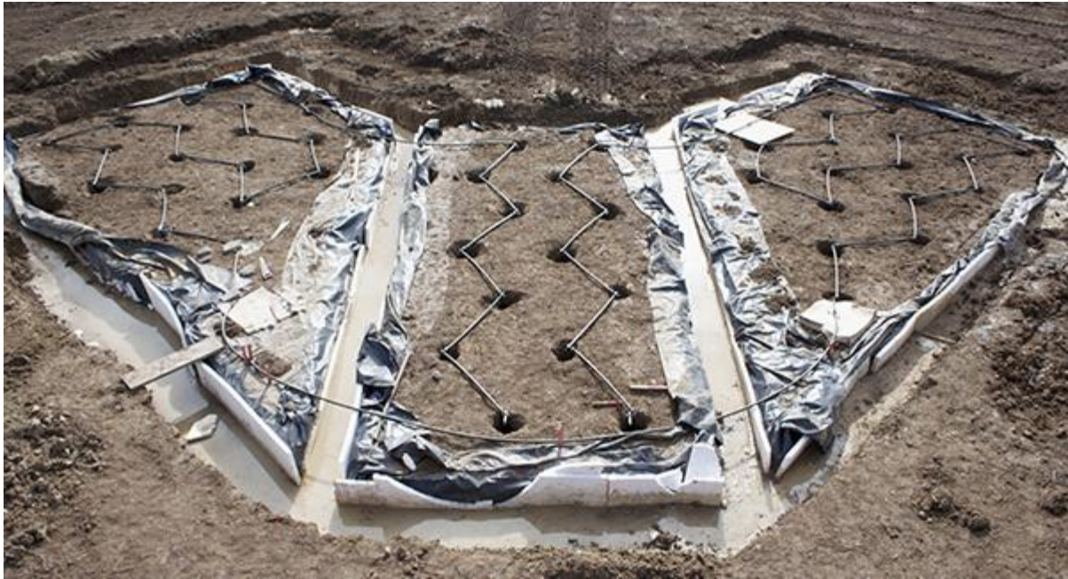
Figure 18 An earth energy bank installed underneath a new build property with PV-T. Image courtesy of Caplin Homes
