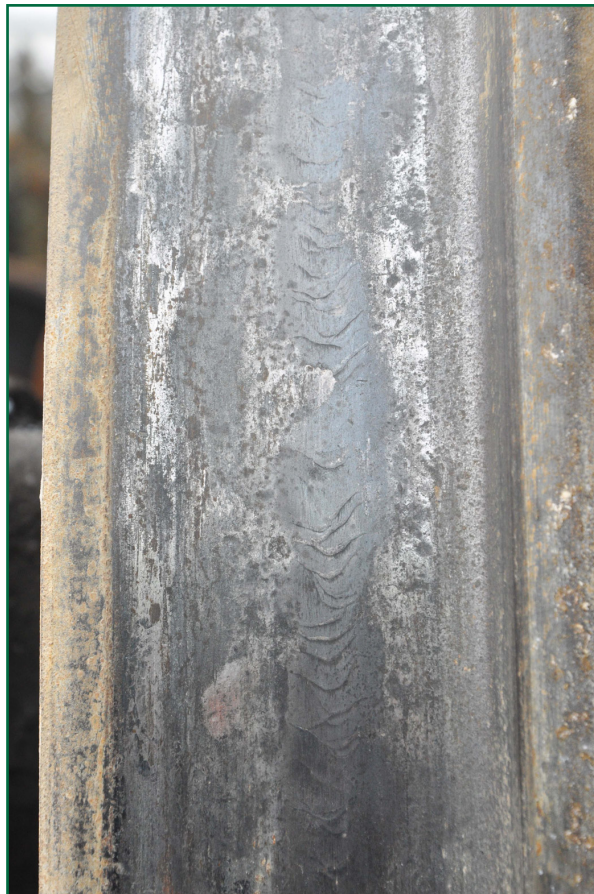
Figure 7: Example of thermal damage to the tread surface (by courtesy of Serco Rail Technical Services)
