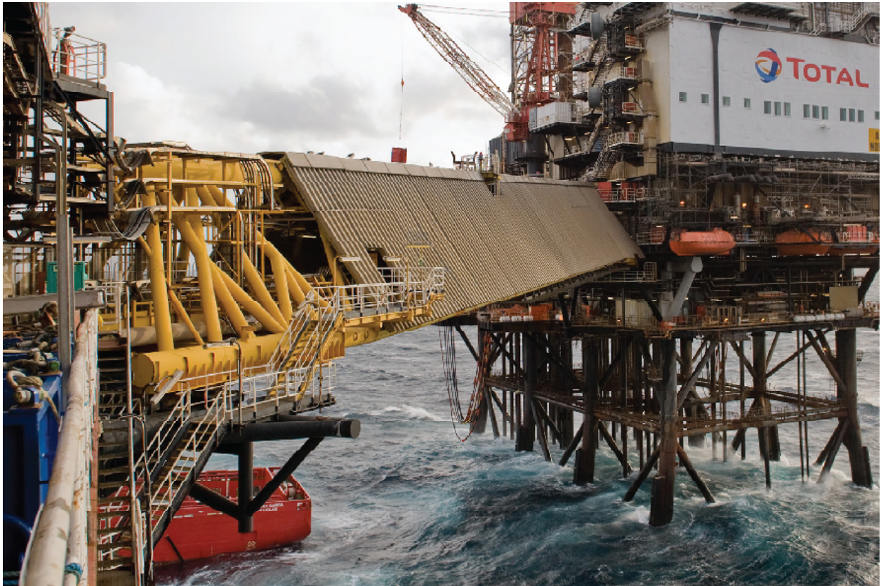
Figure 3 : Alwyn North Platform
