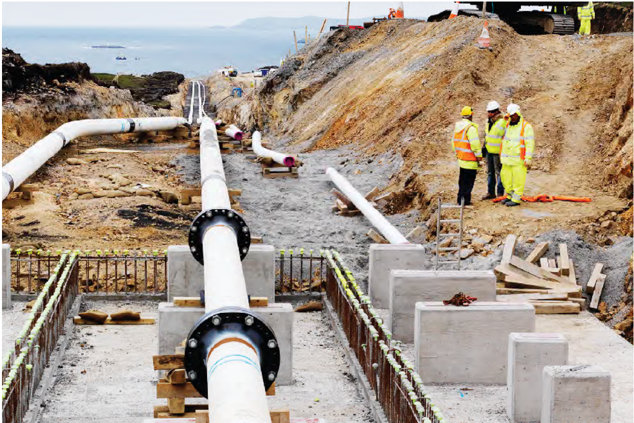
Figure 8 : Shetland Pipeline Infrastructure
