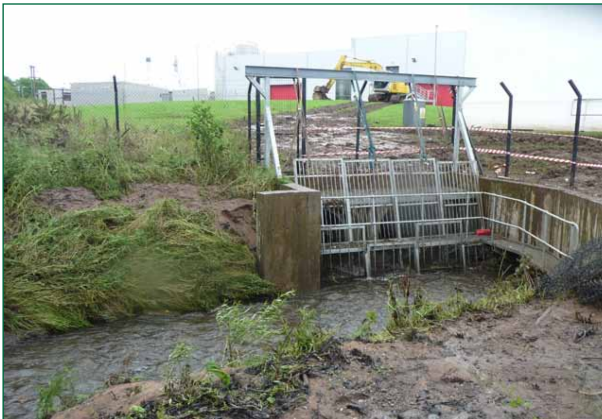
Figure 8: CCHBC culvert inlet with trash screen (image courtesy of URS)
