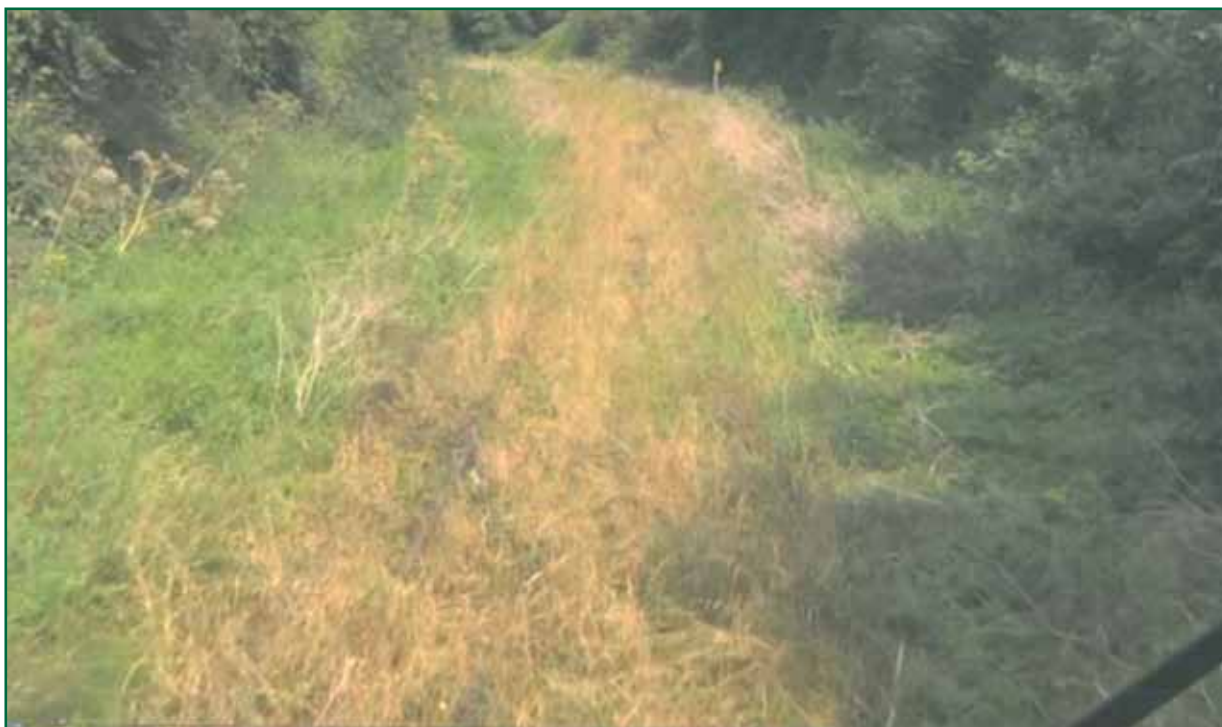
Figure 14: A section of the Antrim branch line with excessive weeds and lack of visibility of the track, September 2012
