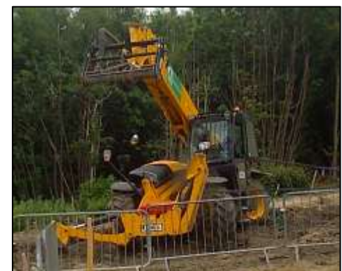
Position of mast and outrigger when FLT was turned upright
