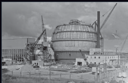
WAGR was built between 1957 and 1961 and was the forerunner to the UK's second generation of power reactors
