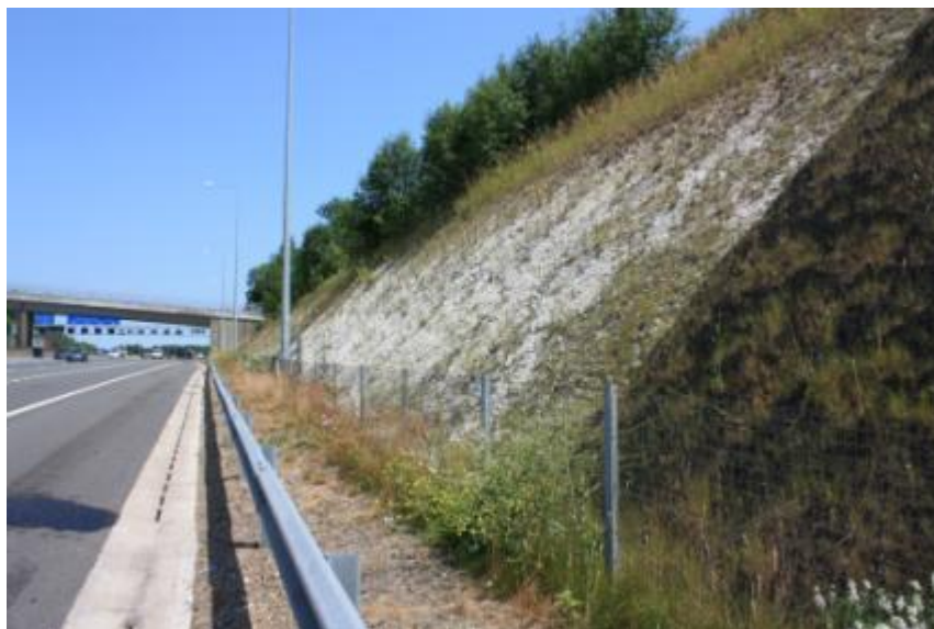
Figure 5-5– Calcareous grassland is establishing by naturalisation on new cut slopes – no direct seeding was undertaken
