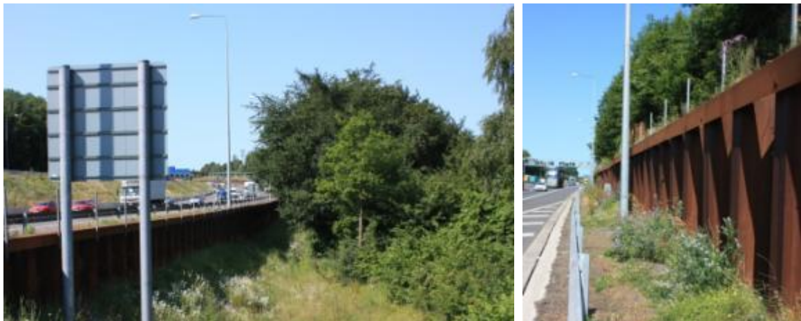
Figure 5-8– Use of sheetpile retaining structures has allowed for the retention of mature vegetation within the Scheme boundary
