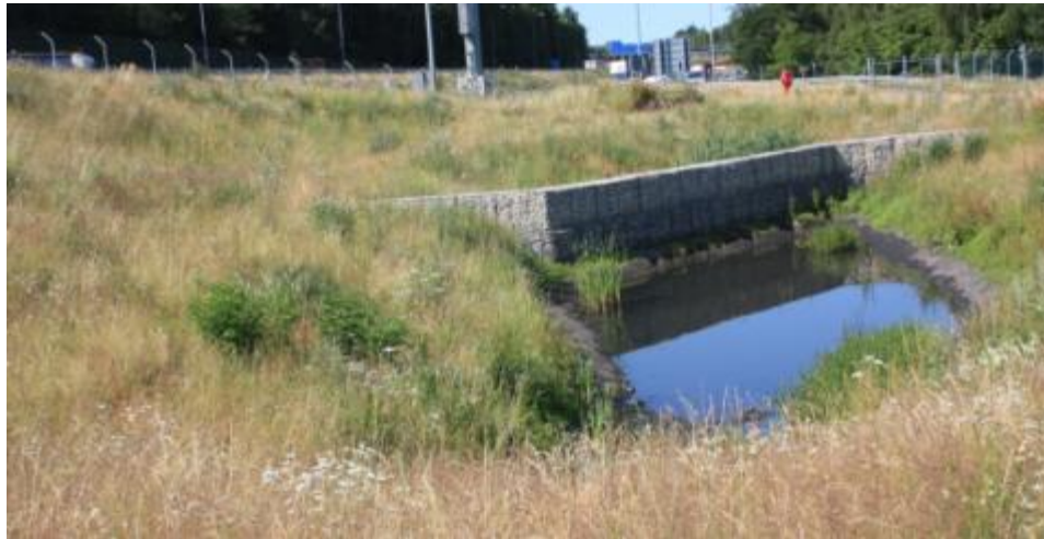
Figure 5-24– Pond 15 between junction 20 and 21
