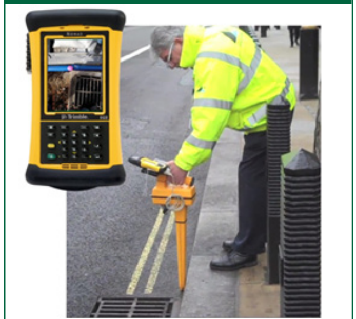
Figure 4 - Photo of exposed duct and RFID tag being accessed from associated tag data
