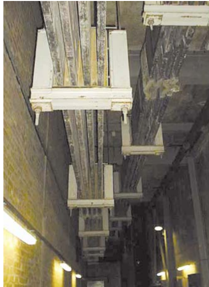
FIGURE 2.3 Power supply bus-bars in the roof of a corridor at a chloralkali plant (courtesy of Ineos Chlor)
