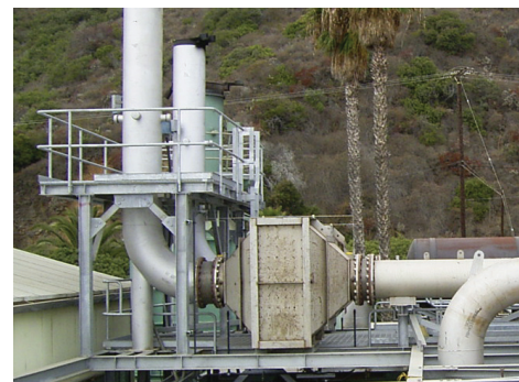
An installed SCR system.
