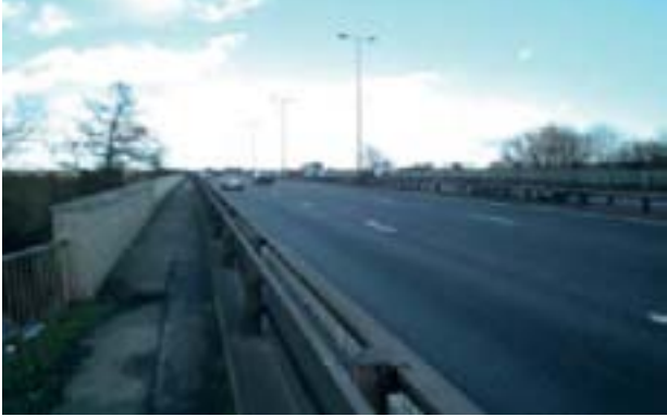
Figure 6: Discontinuous hard shoulder at underbridge
