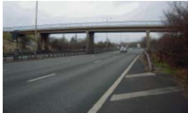
Figure 5: Discontinuous hard shoulder at overbridge
