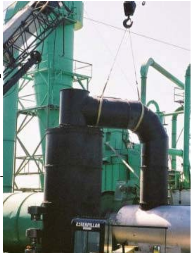
20 MM Btu/hr solid fuel burner for a drying system. Drying system retains capability of using natural gas as a fuel.
