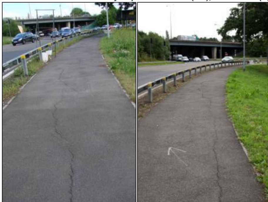
Figure 5-14 – Cracks in the Footway between the M25 Anti-Clockwise Exit Slip Road and the A12 London-bound Entry-Slip Road at OYA (left), and at FYA (right).
