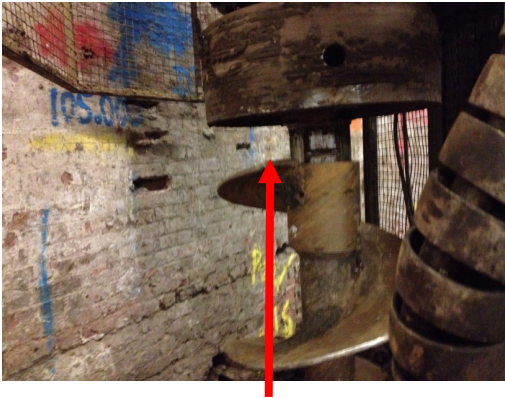
Hand resting on the top flight as duplex lowered onto the next auger
