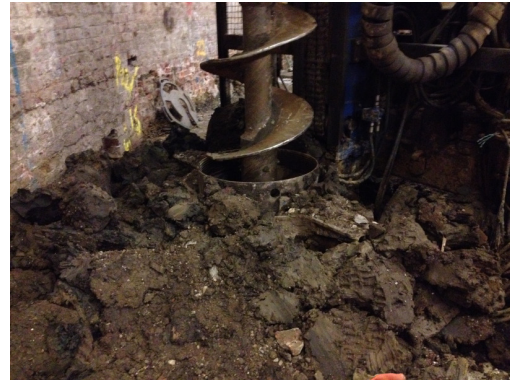
Buildup of spoil leading to uneven ground conditions
