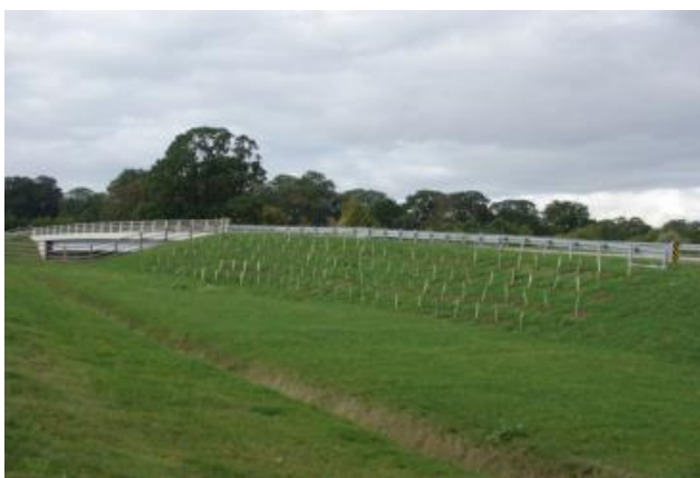
Dead landscape planting on the south-east embankment of Syerston overbridge
