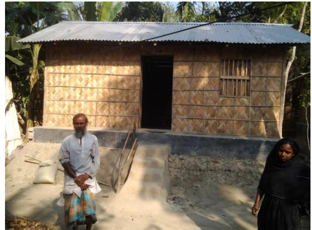
Basic house, back-filling on the base walls, no protection of the screen walls
