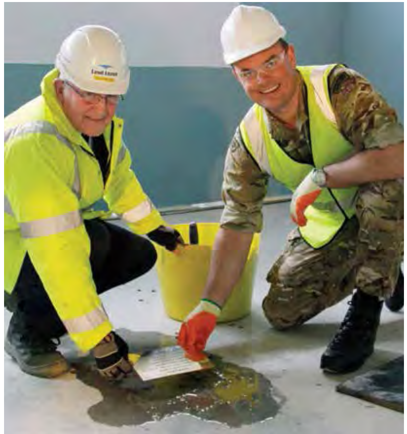
Topping out ceremony of Falklands Building at HMS Nelson , from left, Gwyn Williams and Colonel Mike Tanner
