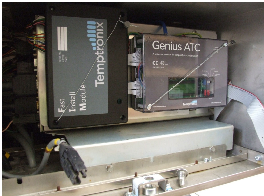
Figure 12 Example of FIM Board
