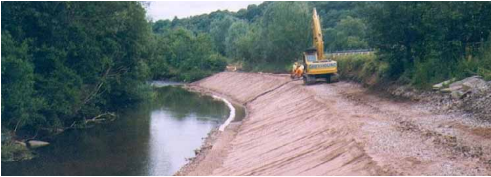
Slope no steeper than 1:2 with hazards or obstructions
