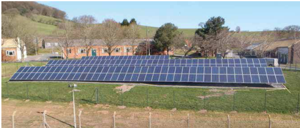
Photovoltaic arrays at Sennybridge Training Camp © Landmarc
