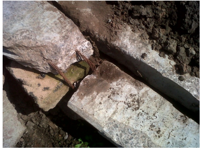
Failed concrete access panel
